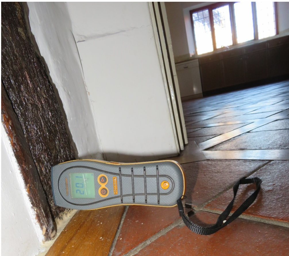
Images 11 & 12: High Masonry Meter Reading (60.9 when 40 is Normal) & Timber Moisture Meter Reading (36% when Under 15% is Normal) – in Kitchen
