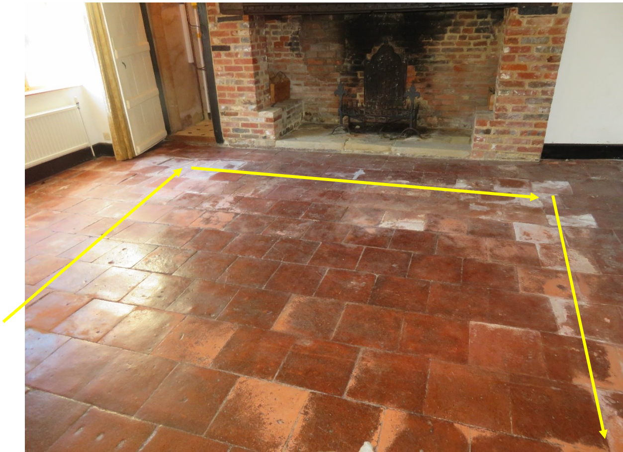
Image 14: Pattern of Salt Efflorescence to within the Reception Hall
