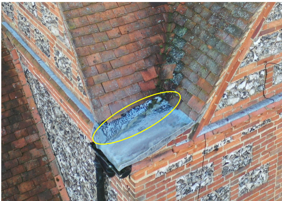
Image 3: High Level of Surface Patina & Past Bitumastic Repairs to Lead
