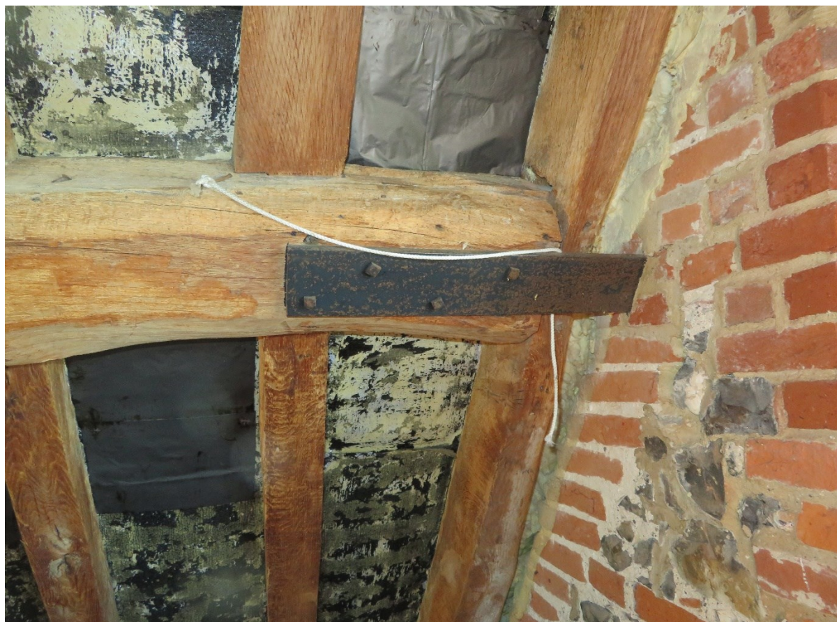
Image 5: Historic Repair to Roof Structure
