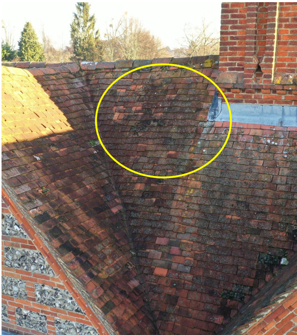
Image 2: Slipped/Slipping Tiles to Front Elevation
