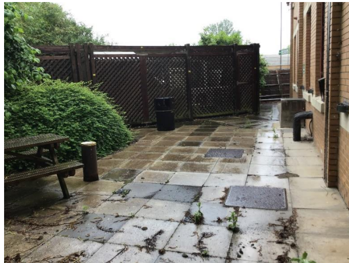
PLATE 2 SHOWING HARDSTANDING PAVING
