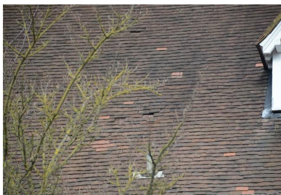
Missing tiles on southern elevation.
