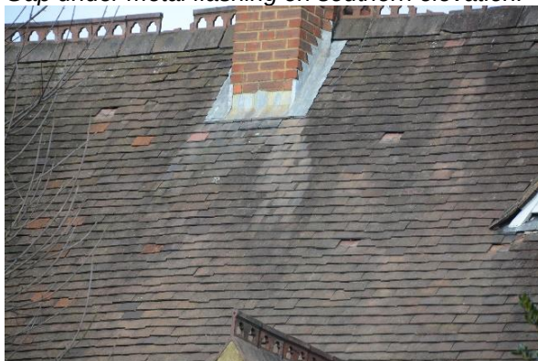
Missing tiles on southern elevation.
