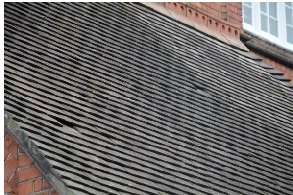
Missing tiles on northern elevation.
