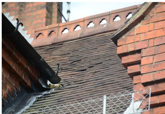
Dislodged tiles on southern elevation.
