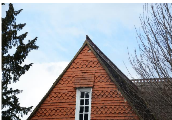
Missing hanging tile on southern elevation.
