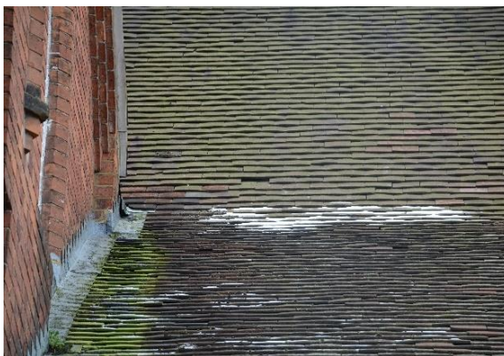
Missing tile on northern elevation.
