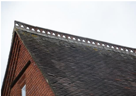
Missing tile on north western elevation.
