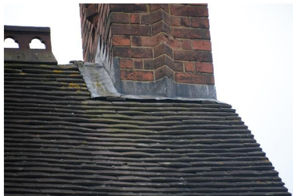
Gap under lead flashing on northern elevation.
