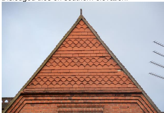
Missing hanging tile on southern elevation.
