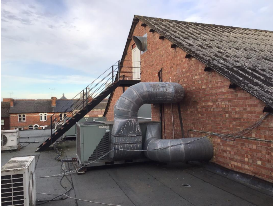
Air conditioning plant.
