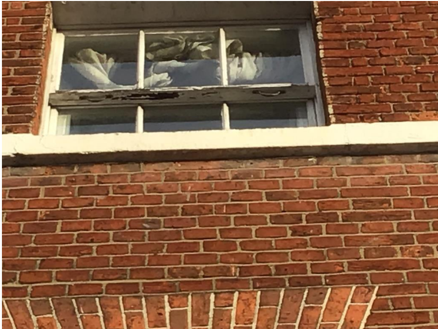
Rotten sash on second floor
