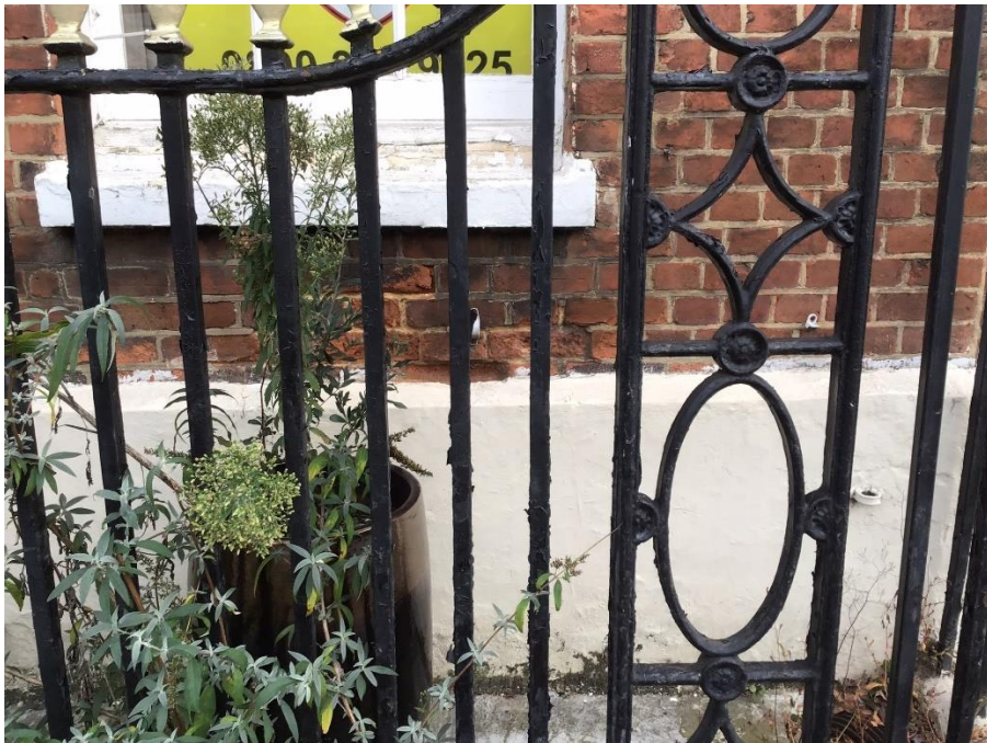
Spalling brickwork above plinth
