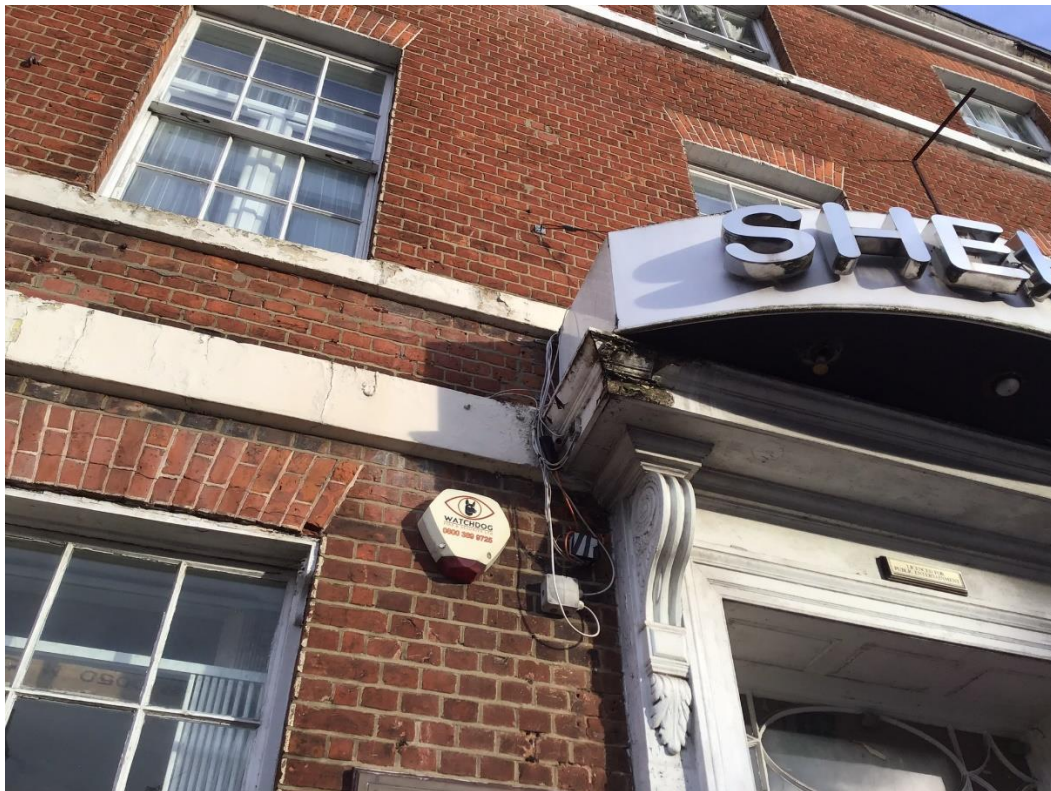
Front canopy, corner rotting
