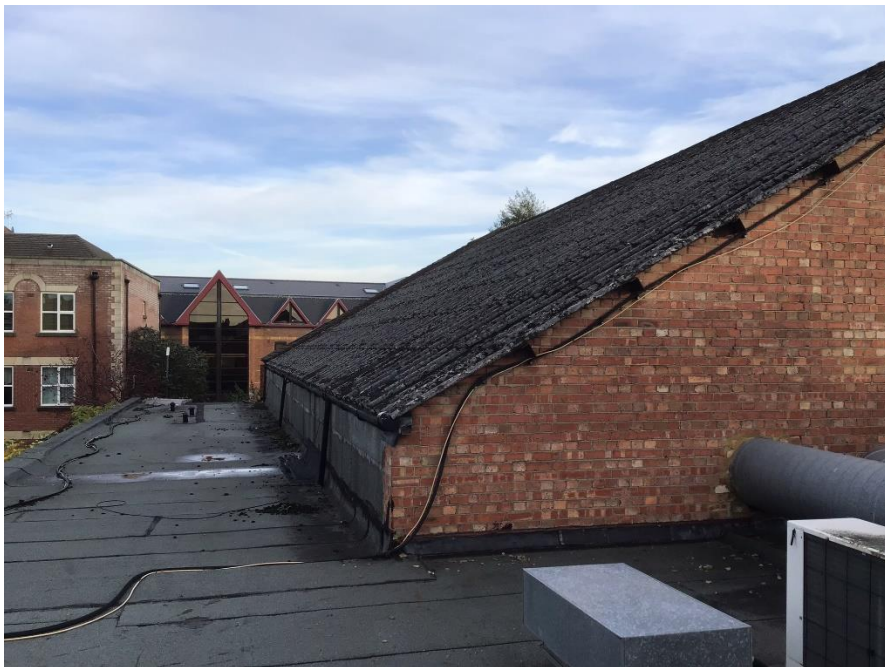
View of corrugated cement, possibility asbestos based roof sheeting.
