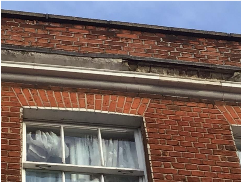
Cornice over second floor windows deteriorating
