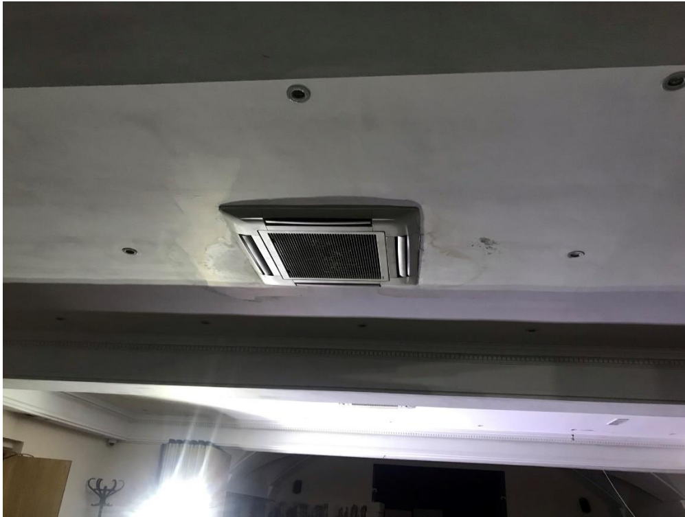
Leaking roof around another a/c unit under flat roof
