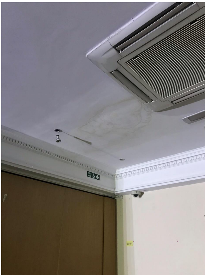
Leaking around another a/c unit under flat roof
