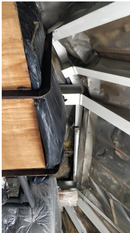
Photo 4: Interior of plant room
