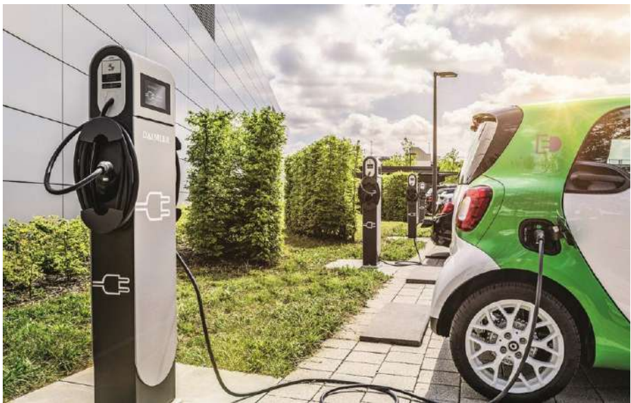
Electric charging facilities
