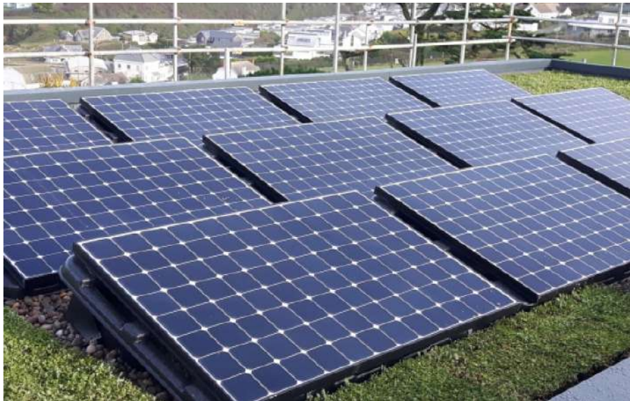
Rooftop PV panels
