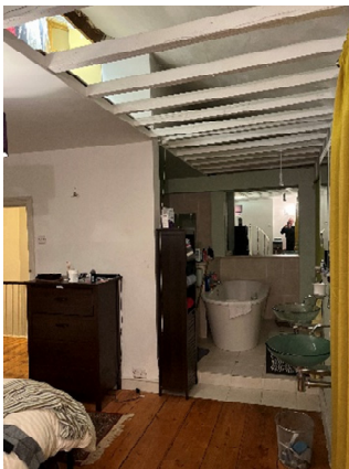
Photograph: 8 Level: First Floor View: From Bedroom 1 into Ensuite Element: Area to be closed up
