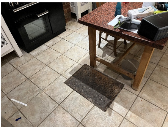
Photograph: 5 Level: Basement View: Inspection chamber and cover within kitchen Element: Inspection chamber and cover to be removed
