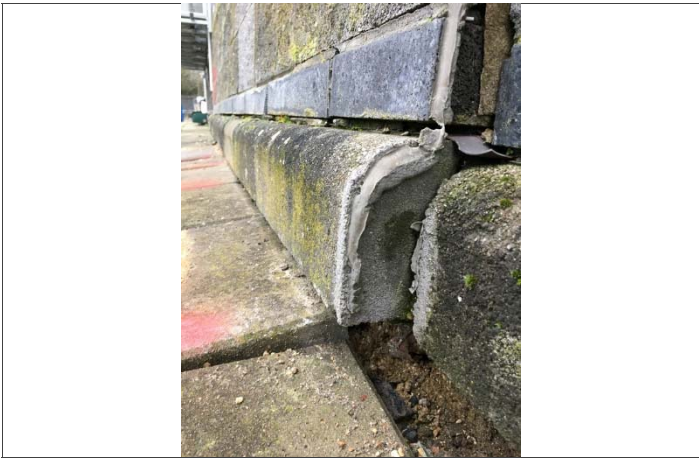
07: Section of damaged wall
