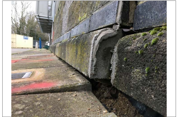
10: Section of damaged wall
