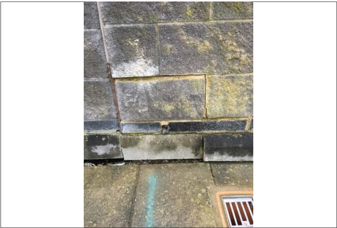
08: Section of damaged wall
