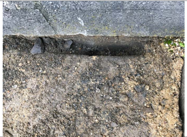
14: Gap between concrete and wall
