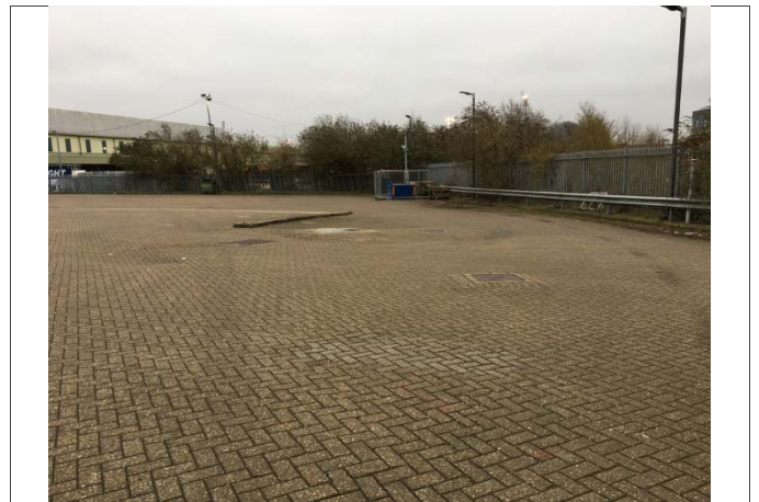
12: Uneven ground surface
