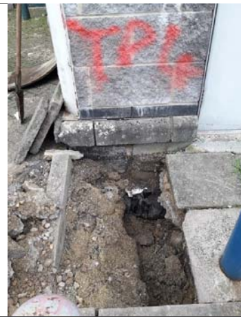
16: Broken through concrete beam
