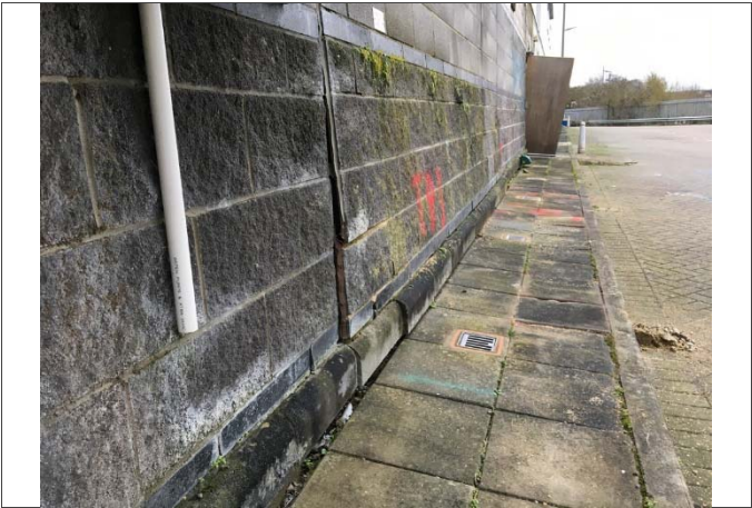
06: Section of damaged wall
