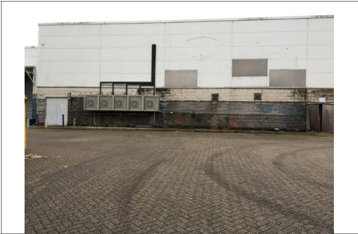
05: Section of damaged wall
