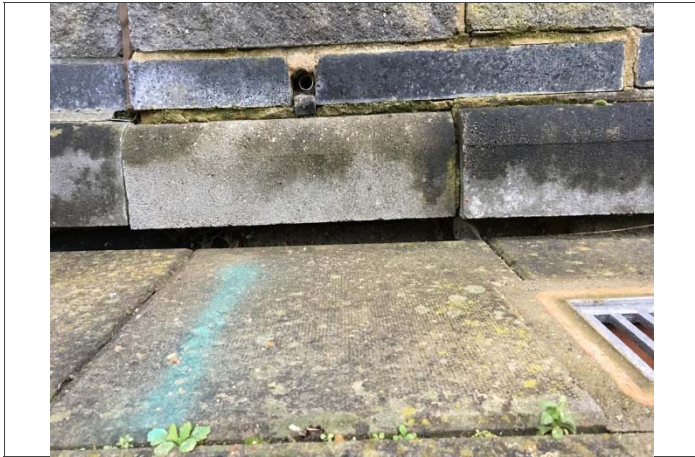
09: Section of damaged wall
