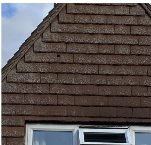
Photo 7: Close up of the hanging tiles on the rear elevation of the building showing a potential roost access point
