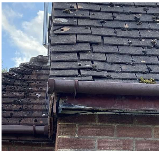
Photo 5: Close-up of loose roof tiles on the east side of the building
