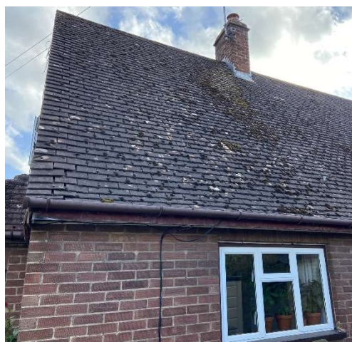
Photo 4: Tiled roof on the east side of the building shown some loose tiles on the lower left-hand side
