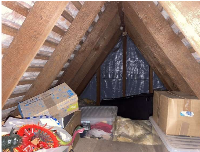
Photo 9: The northern part of the loft void, showing absence of lining beneath the tiles
