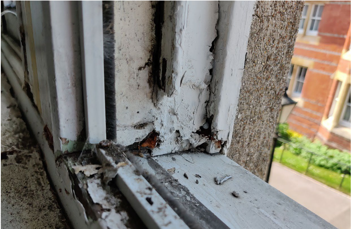
Figure 13. Parting bead missing, weight pocket painted in, front cheek of sash box damaged.
