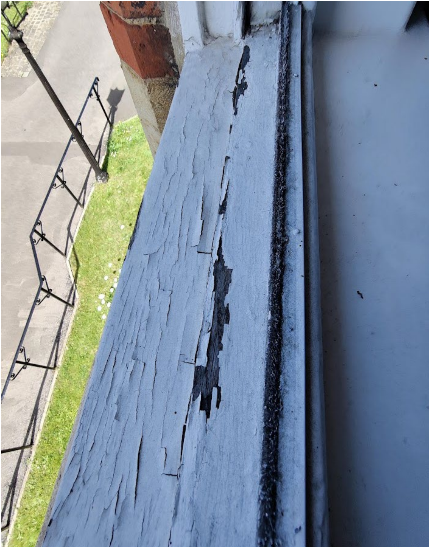
Figure 12. Cill at first floor level, less regularly painted, wood exposed and starting to rot.
