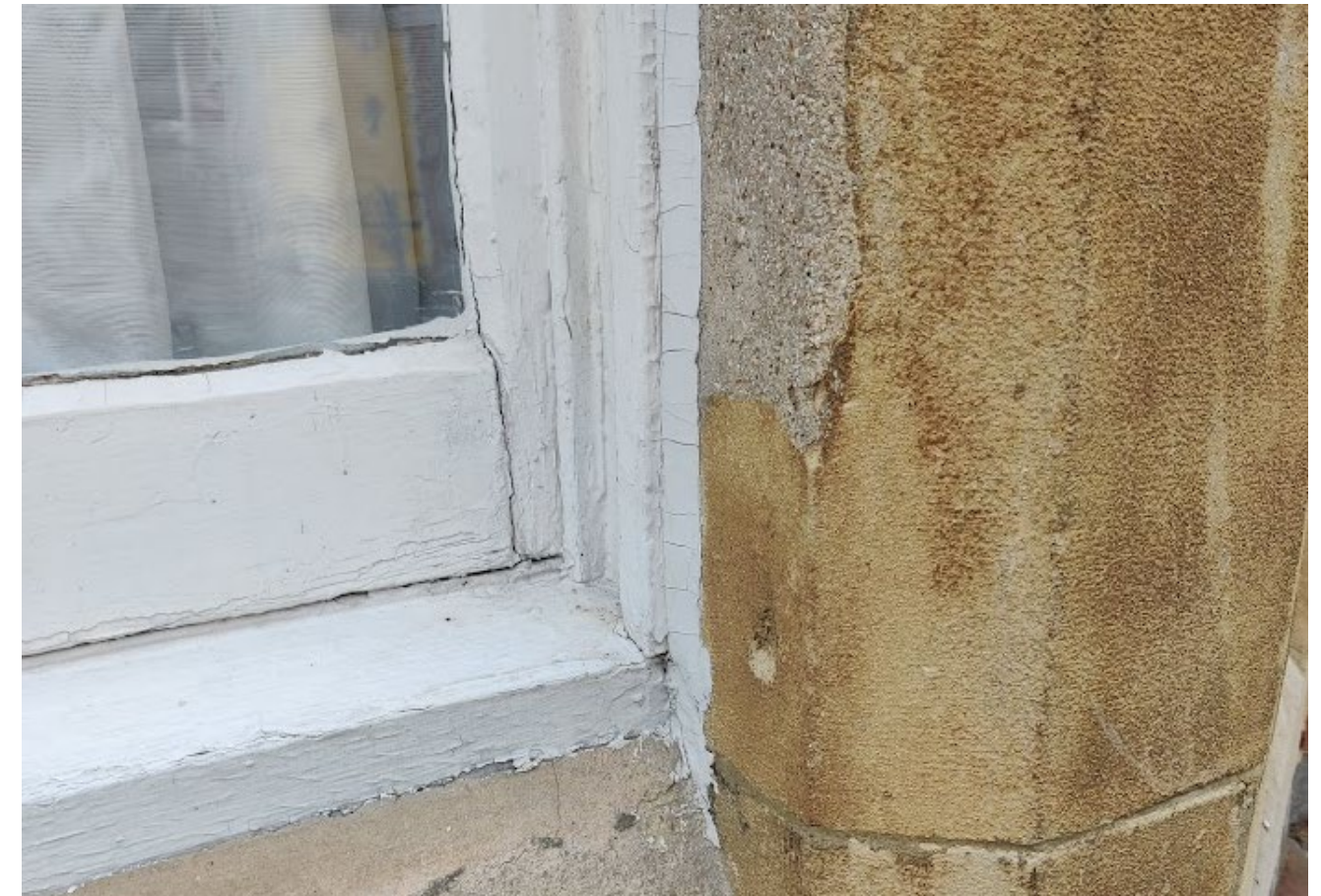
Figure 8. Typical Joint Opening Up in Lower Sash Frame
