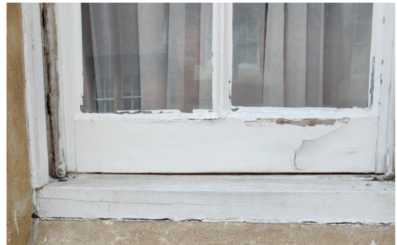
Figure 10. Pulley Linings and Parting Beads in poor condition. Paint peeling away.
