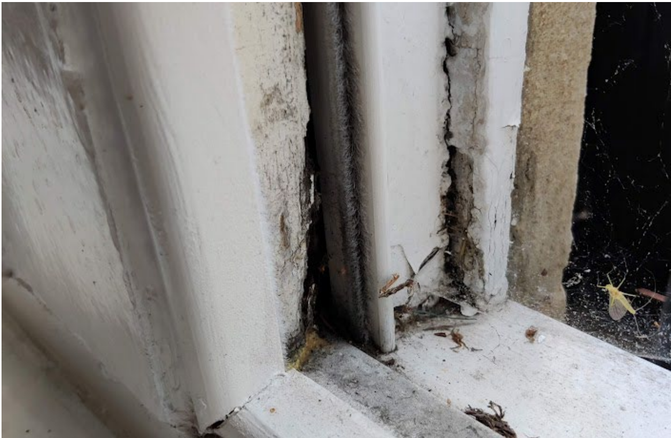
Figure 11. Parting bead and weight pocket junction damaged and in need of repair. Front cheek of sash box starting to rot at base.
