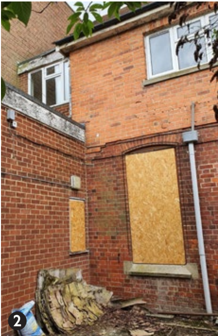
Condition of extensions to rear
