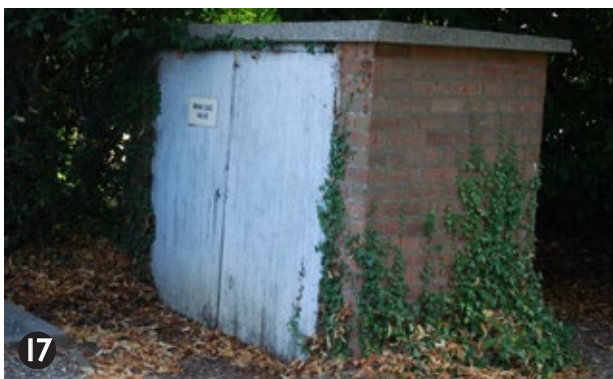
Gas valve at the south-west corner of the site
