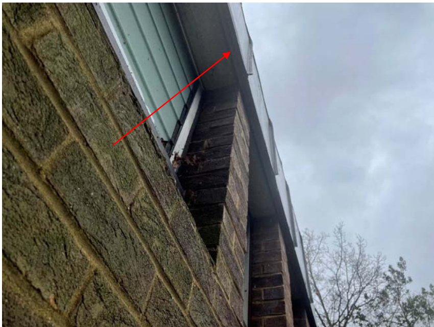
Plate 1 Gap behind overhang of lead cladding, single storey Changing Rooms
