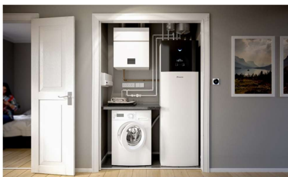
Figure 5, Typical HIU Packaged Utility Room
