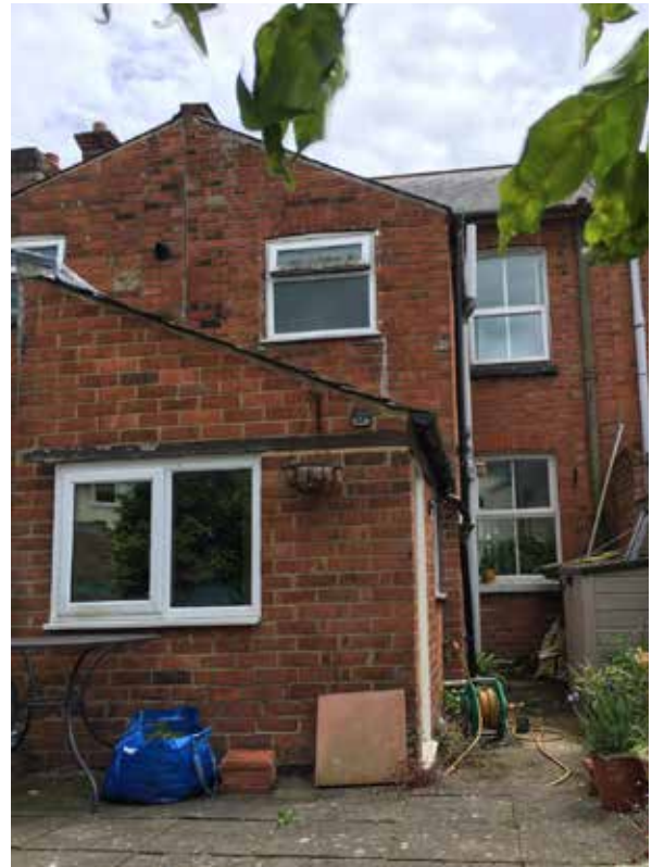
Figure 5: Photograph of poorly constructed original rear extension with mono pitch roof.
