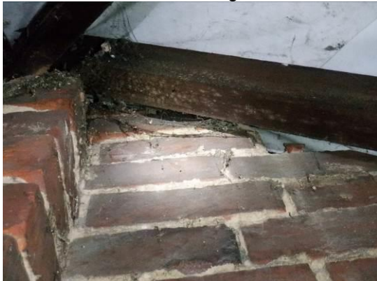
17. Party end wall of single-skinned brick construction with gaps around the edges.
