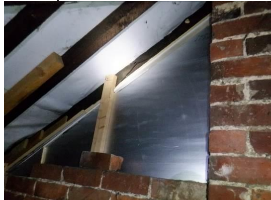
18. Missing brickwork at party end wall with insulation boards behind.
