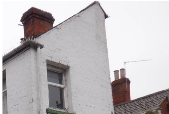
4. Gaps under verge tiles at the western end of the house.
