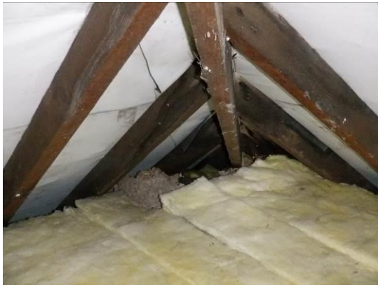
19. Wasp's nest present in the north-eastern corner of the roof space.
