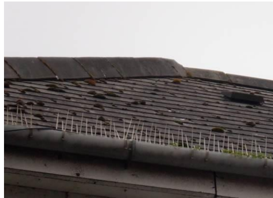
6. Occasional lifted hip tiles.
