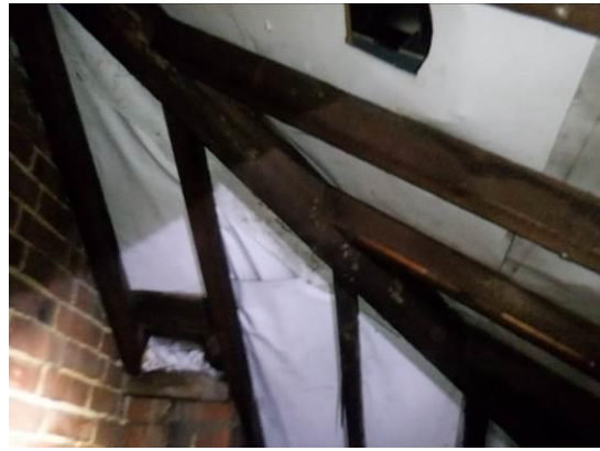
14. Gap in breathable roofing membrane around a vent.
