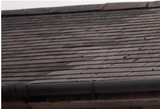
3. Slate tiles mostly flat and tight across the roof.
