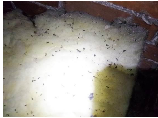
20. Accumulation of small-sized bat droppings on the insulation at the base of the party wall.
