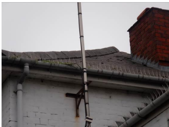
7. No mortar visible under hip tiles at the western end of the building.
