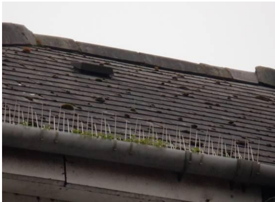
5. Gaps under the ridge tiles along the southern side of the roof.
