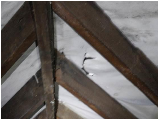
15. Tear in breathable roofing membrane.
