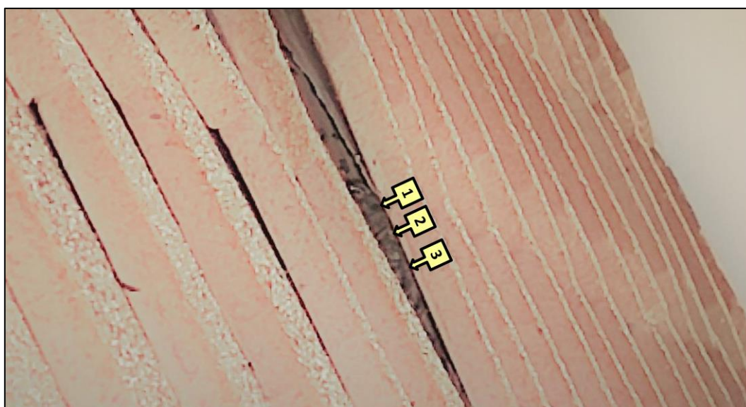
Figure 6 – 3x Pipistrelle spp. bats roosting in the batten space behind the lifted hanging tile on the rear elevation at 16 Tower Close
