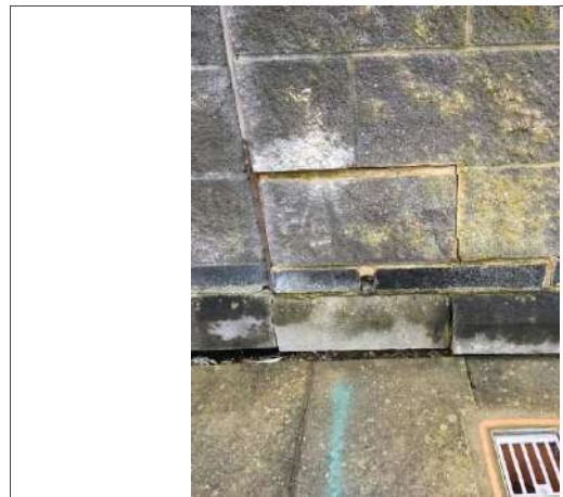
08: Section of damaged wall
