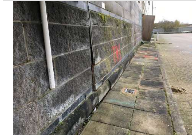
06: Section of damaged wall
