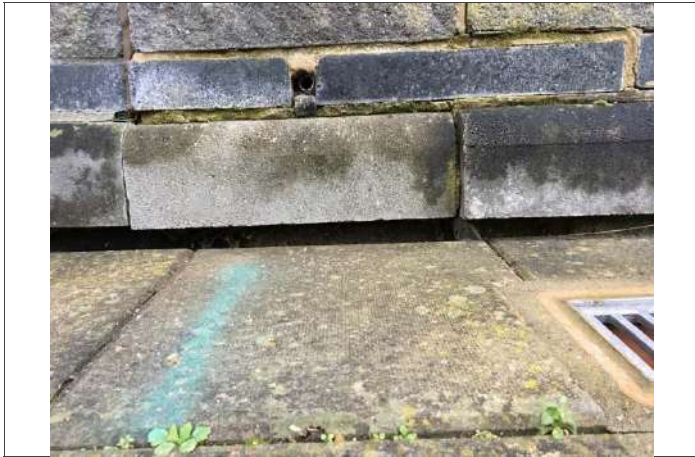
09: Section of damaged wall
