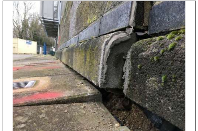
10: Section of damaged wall
