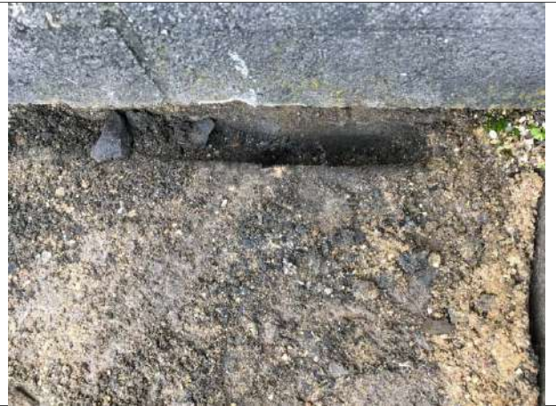
14: Gap between concrete and wall
