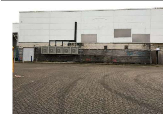
05: Section of damaged wall
