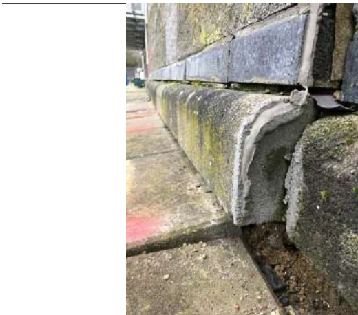
07: Section of damaged wall
