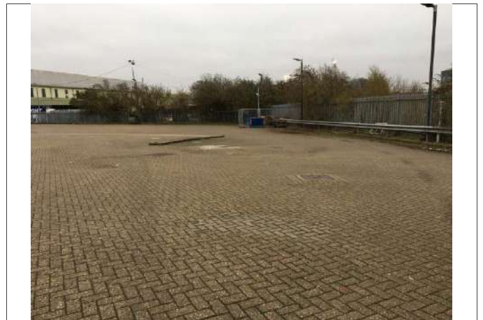
12: Uneven ground surface
