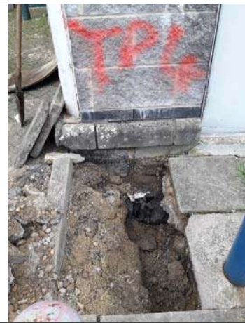
16: Broken through concrete beam
