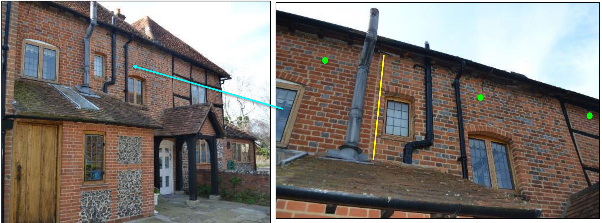
Figure 19: Details of east elevation-the variation in brick work along this elevation suggests contemporary alterations- it is clear that the first floor brick work can be divided into three distinct sections (highlighted in green), the central section does not tie into the neighbouring section suggesting a late 20 th /21 st century alteration/repair-possibly when the windows were altered (highlighted in yellow)
