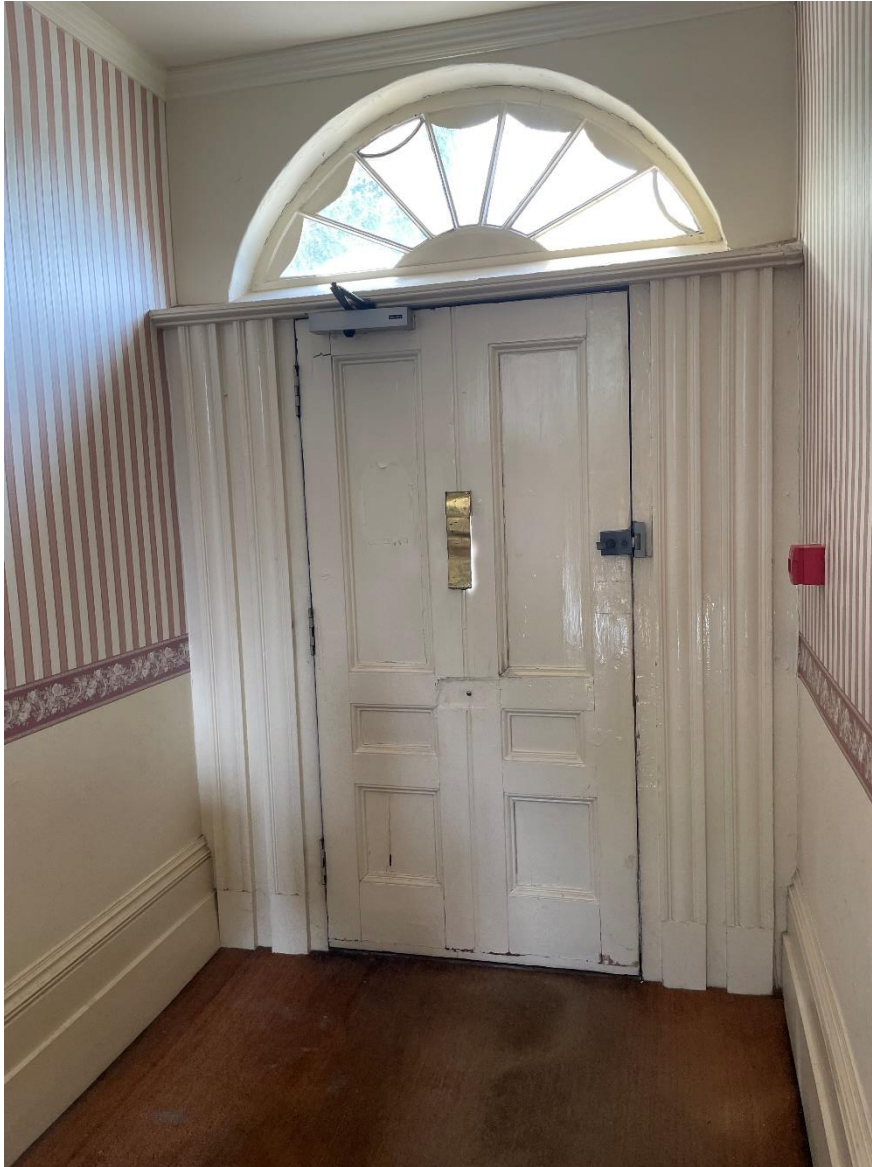
Photograph 1: Main entrance door unit. Note existing unit and fabric is to be retained. There is no proposed alteration in style as part of refurbishment and redecoration. The current poorly fitted letterbox is to be replaced with an intumescent unit and internal door furniture only is to be replaced to maintain a uniform aged brass finish.
