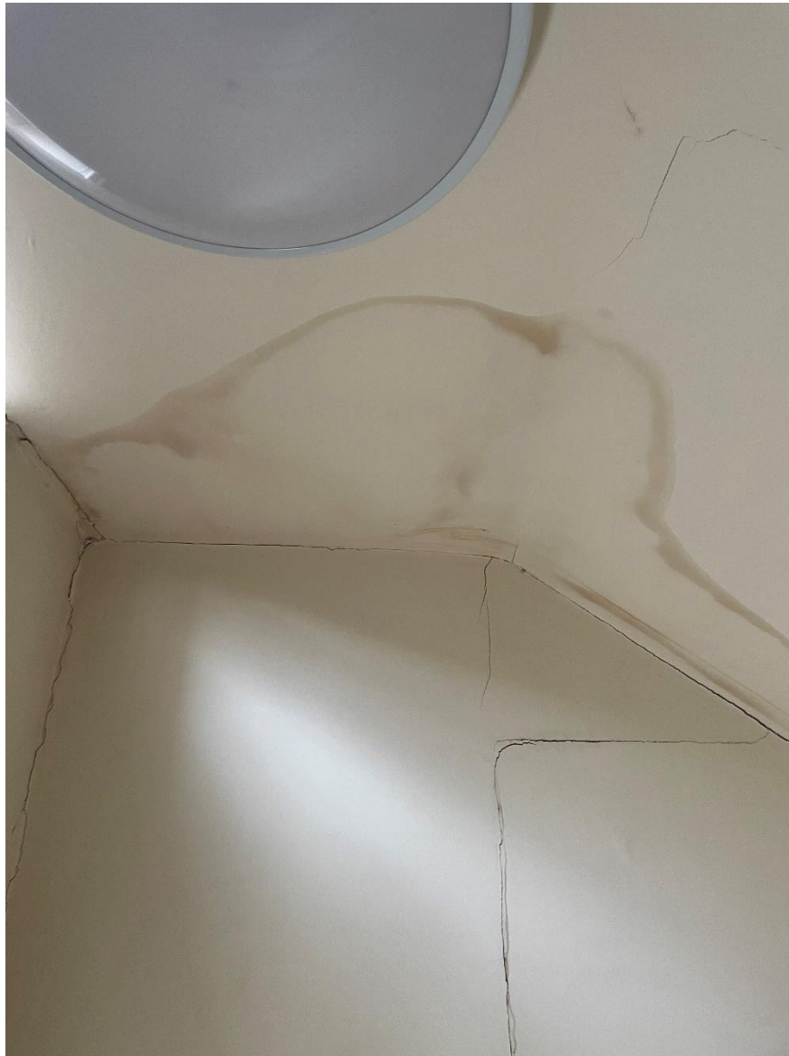
Photograph 9: Existing cracking across current plasterboard finishes and staining as a result of historic water ingress. External defects have been previously rectified. Localised replacement of plasterboard finishes is proposed where de-bonded or failed.
