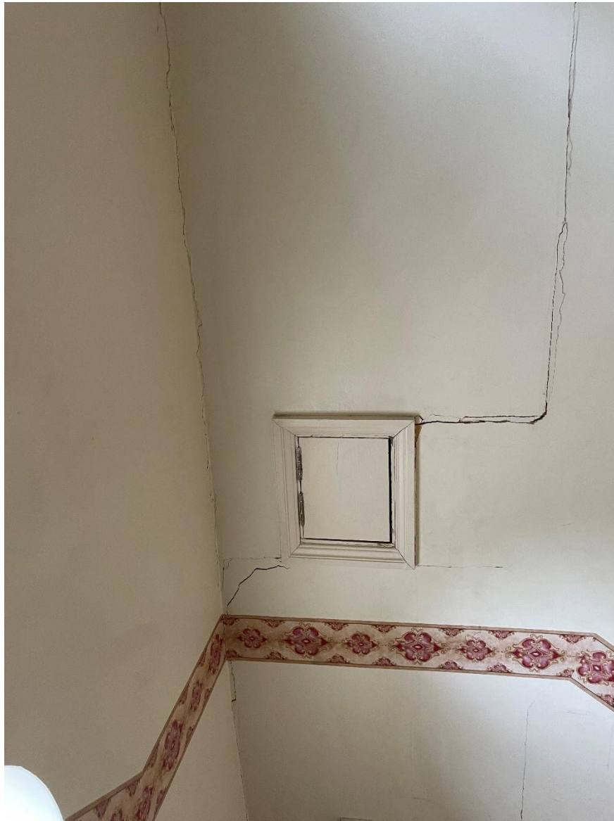
Photograph 8: Riser cupboard access hatch and existing cracking defect within adjacent plasterboard finishes. Proposed works are to remove the access hatch unit and install fire-rated replacement flush with wall finishes, and to replace localise plasterboard finishes only where failed or de-bonded.
