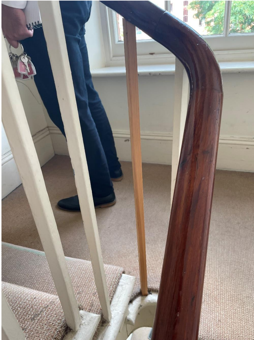
Photograph 7: Missing balustrade spindle to staircase. Repair to match existing adjacent.
