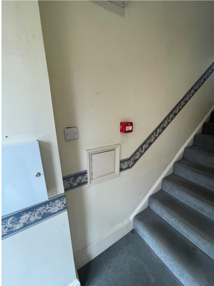
Photograph 4: Riser cupboard access hatch, current wall fixtures and alarm without emergency use signage. Proposed works comprise the replacement of the riser cupboard access door with a fire-rated replacement flush with the adjacent plasterboard finishes. The existing key-cupboard and electrical cover are to be replaced with aged brass fixtures to maintain uniformity in finish.
