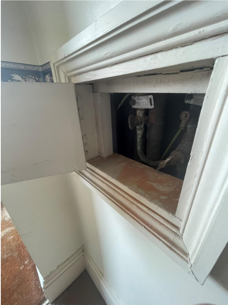
Photograph 5: Showing existing form of riser cupboard access hatch and exposed void.
