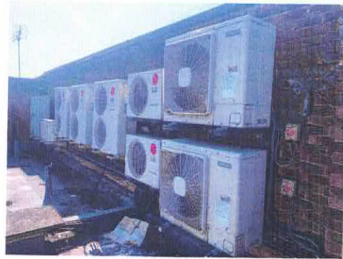
Fig 8: Existing condensers on the roof of the subject building, all to be removed
