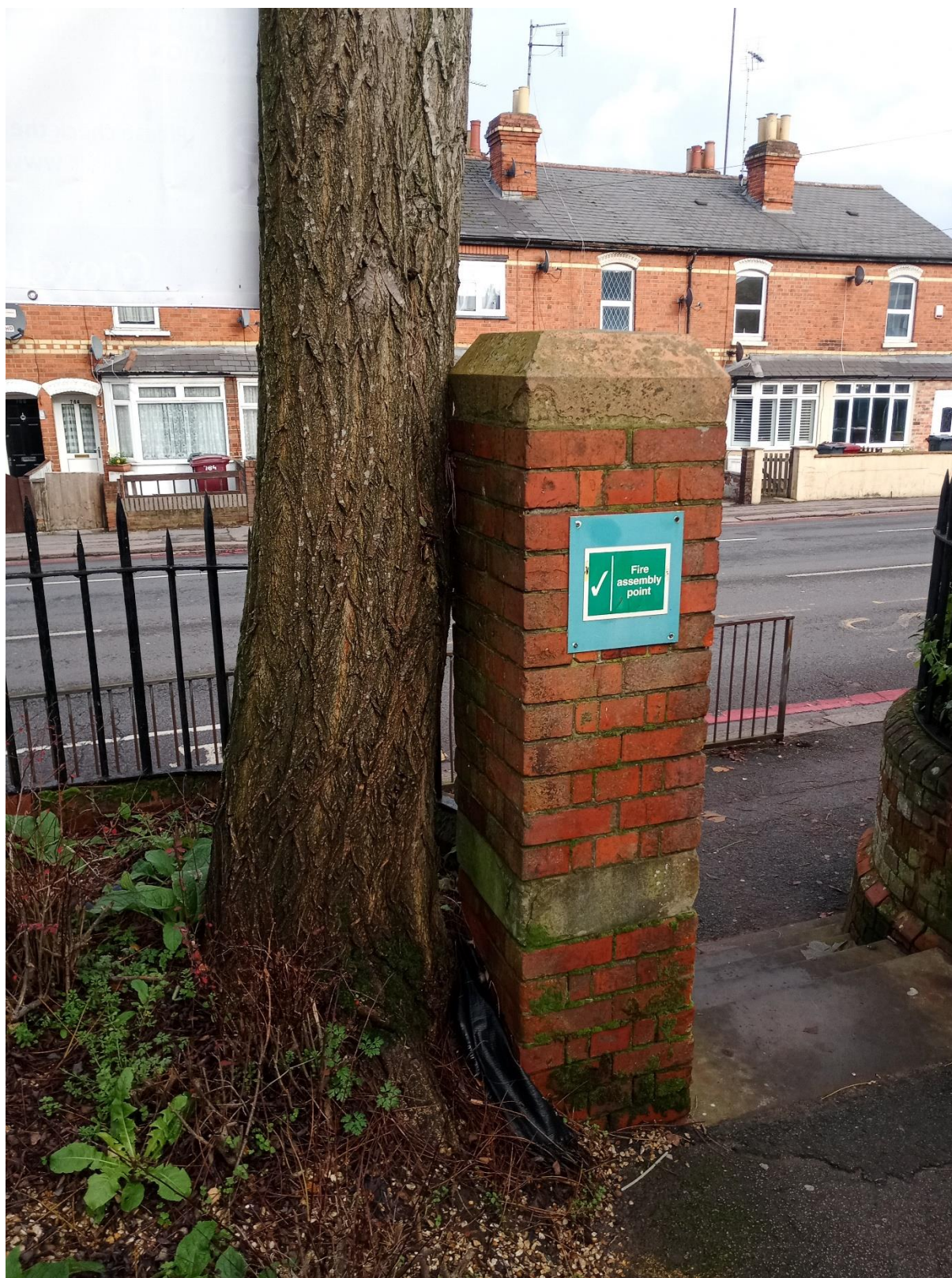
T6 – Growing against brick pillar.
