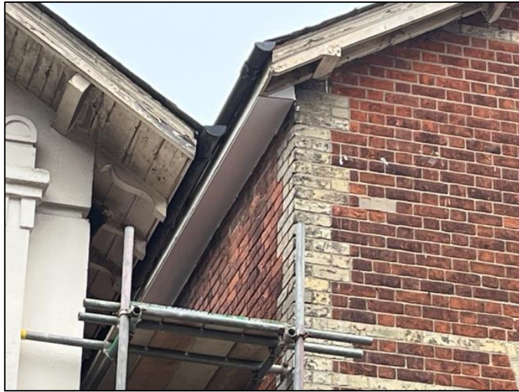
Photograph H Further sealed soffit box with no access for bats
