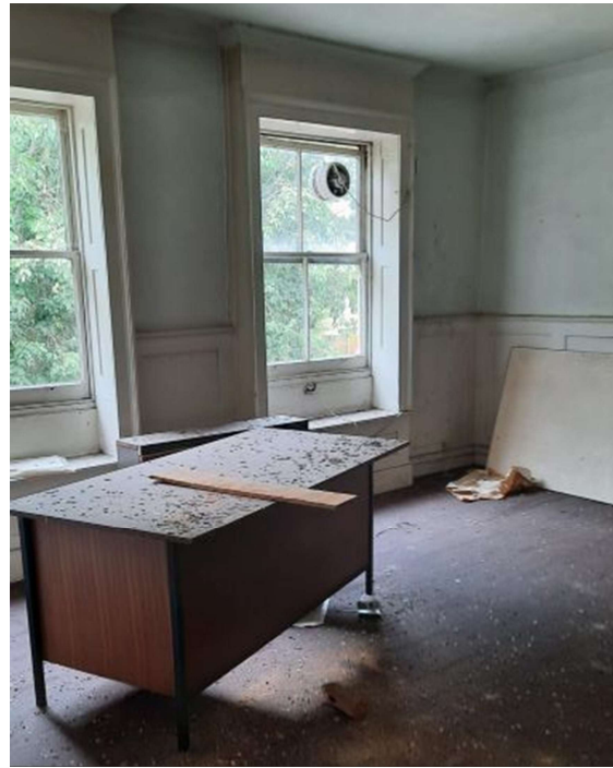
Picture 4: Gap at top of window frame on second floor north elevation.
