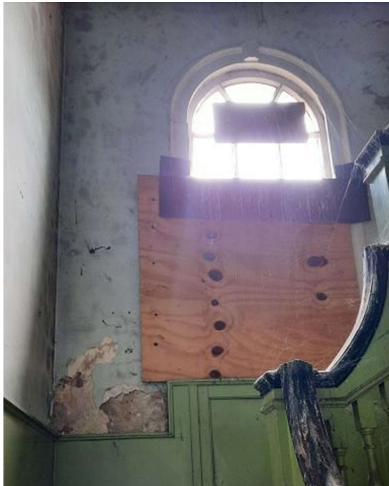
Picture 3: Partially boarded window in stairwell with missing panes behind.
