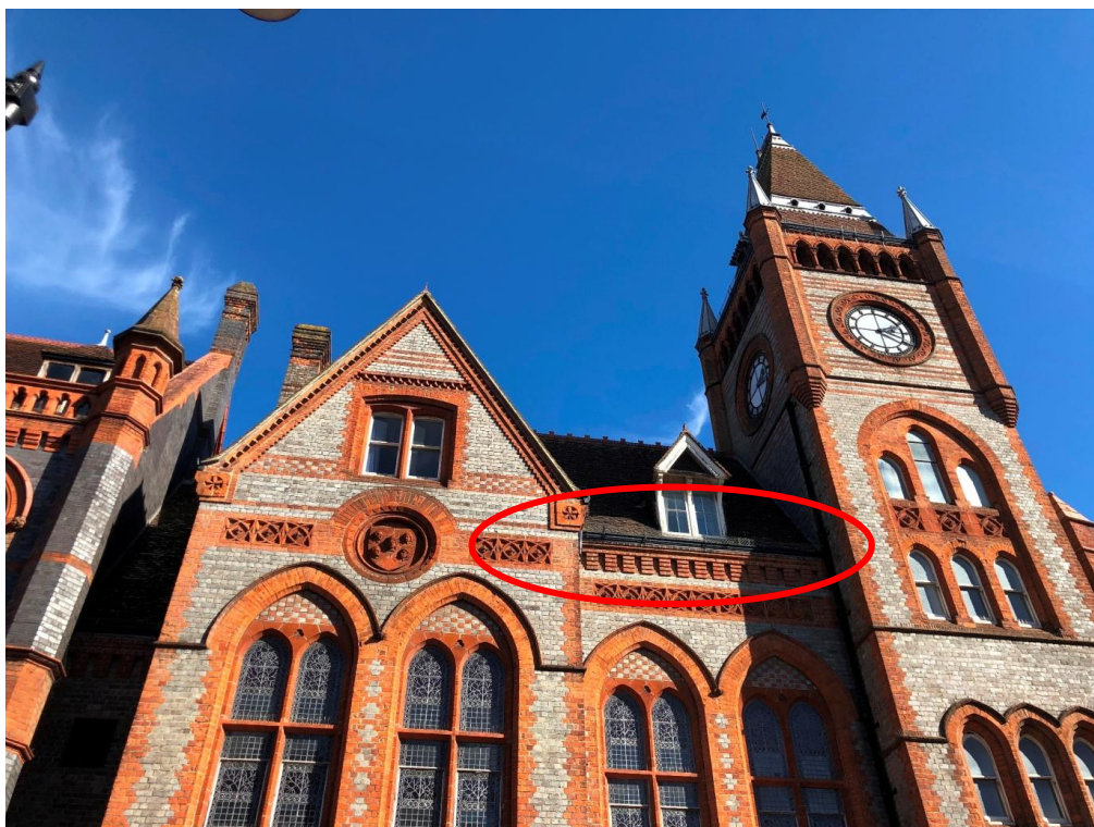
Fig 4: Tile guards fitted to the eaves of Reading Town Hall and Museum
