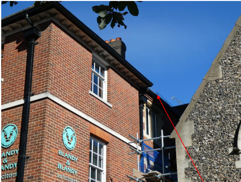
Fig 3: Close up of eaves of adjacent property to the north of the church showing tile guards
