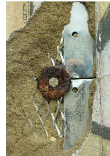
Edge of EML and corroded washers
