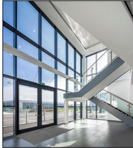
Curtain walling (Internal)
