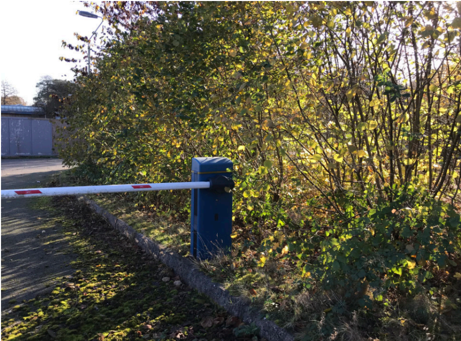
View of site screening trees next to sub-station
