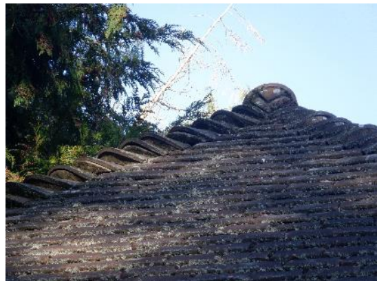
6. Gaps under hip tiles (rear elevation).
