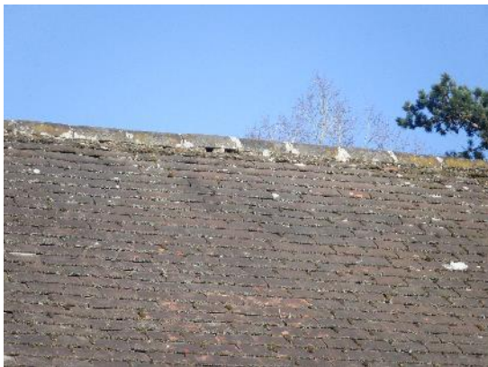
5. Gap below ridge tile (rear elevation).
