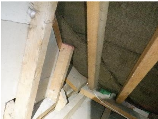
17. Daylight visible at the eaves adjacent to the gable.
