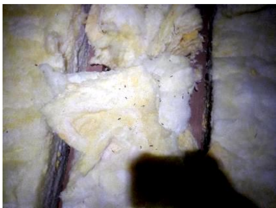
19. Pile of medium-sized bat droppings below ridge at the southern end of the void .
