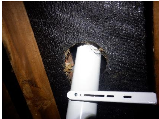
12. Loose roofing felt around flue pipe.
