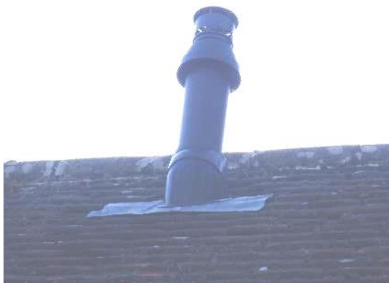
7. Lifted lead flashing around flue pipe (front elevation).
