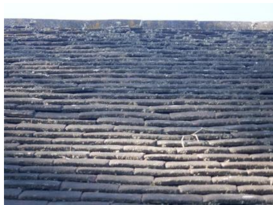
4. Uneven clay roof tiles (southern elevation).
