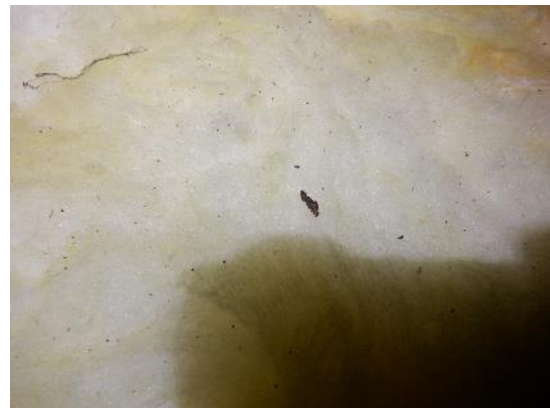
18. Medium-sized bat dropping on fibreglass adjacent to the loft hatch.
