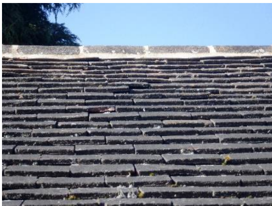
3. Uneven clay roof tiles (eastern elevation).
