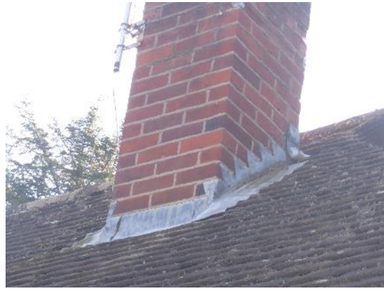
8. Lifted lead flashing around base of chimney (front elevation).
