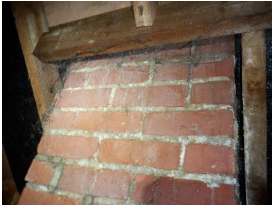
15. Roofing felt tight to cobwebbed brickwork chimney.
