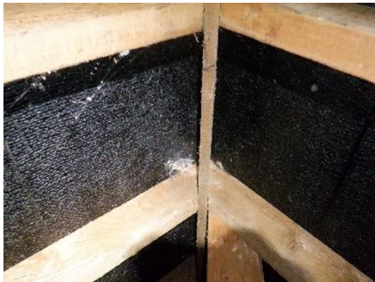
11. Gap in roofing felt beside the ridge at the southern end of the void.
