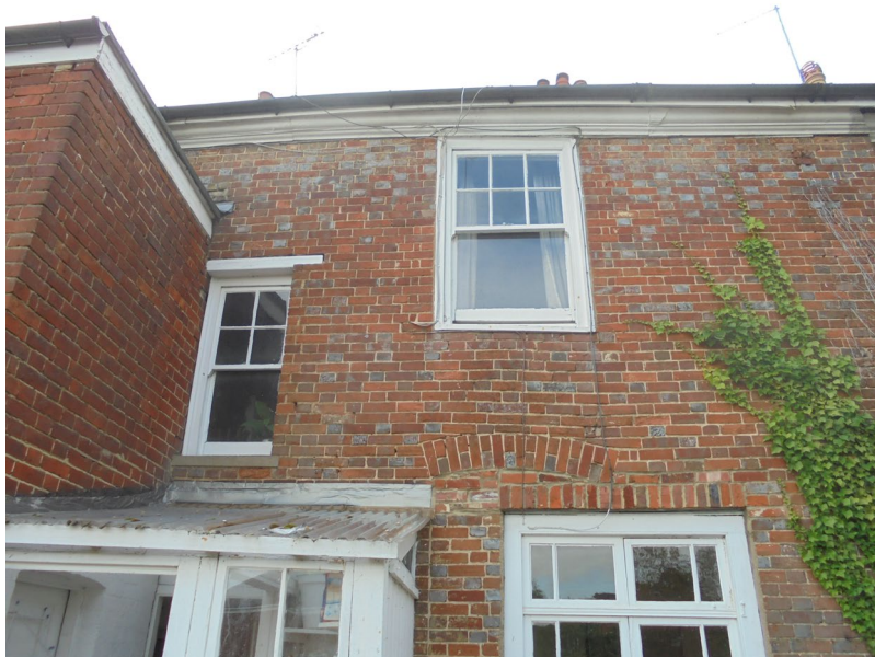
Photo 6 – Photo illustrating the damage to the first floor window
