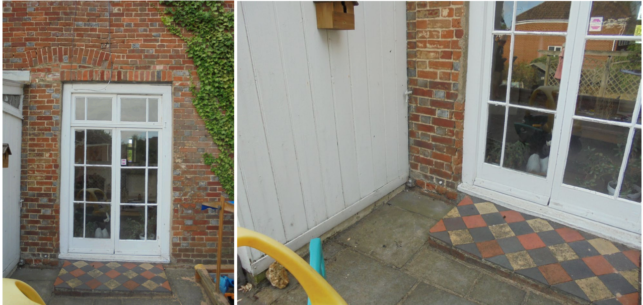
Photo 4-5 – Photos illustrating the damage to the rear door
