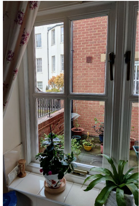
Figure 13. Thick and intrusive glazing bars of existing windows. (Source: Bridges Associates)
