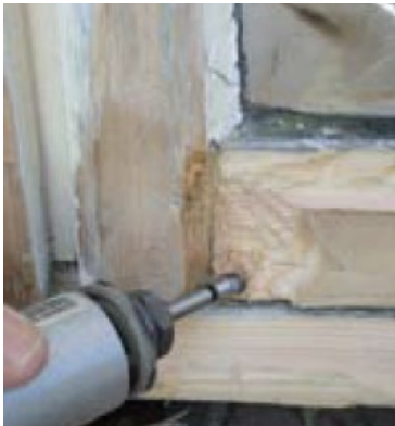
Figure 3. Decayed timber can be removed with a small handheld power tool. (Source: Repair Care International)
