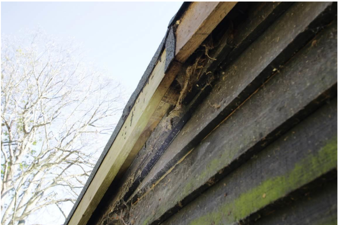
Photo 14: Externally the wooden cladding had occasional gaps and at the rear apex, however limited space in the gaps for bats
