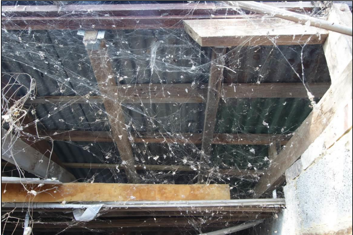
Photo 17: Extensive cobwebs in some of open space of the sheds suggests no recent use internally in the main shed space
