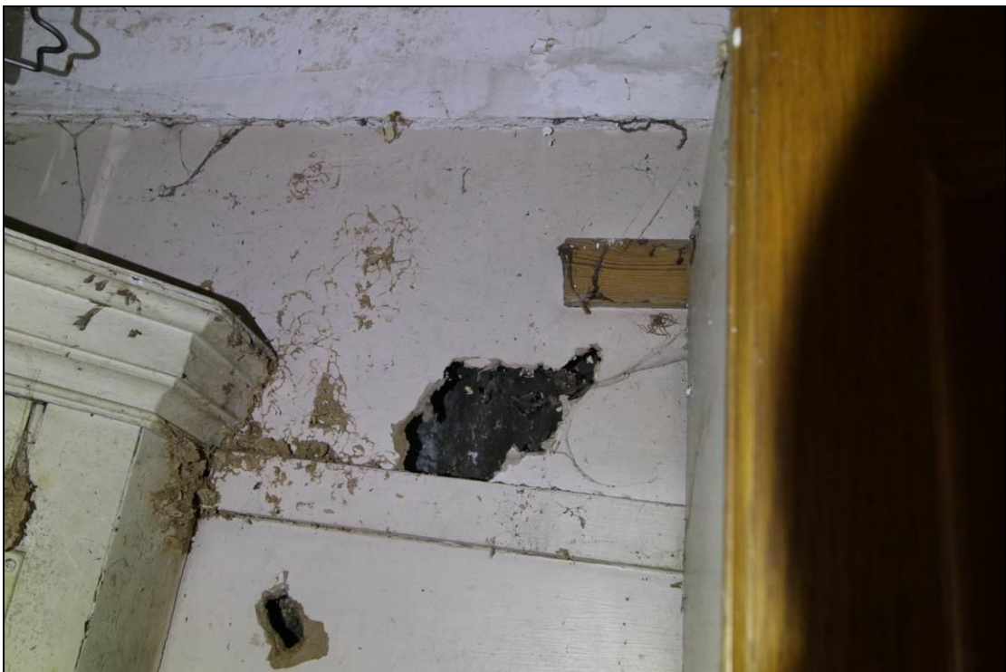
Photo 18: Hole in internal cladding showing small gap, which has been patched up by corrugated metal
