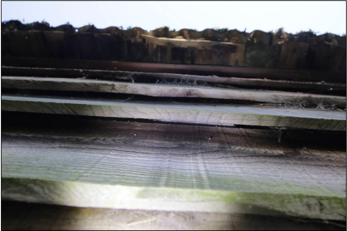
Photo 21: Gap in cladding leading to small void space with some roosting potential.
