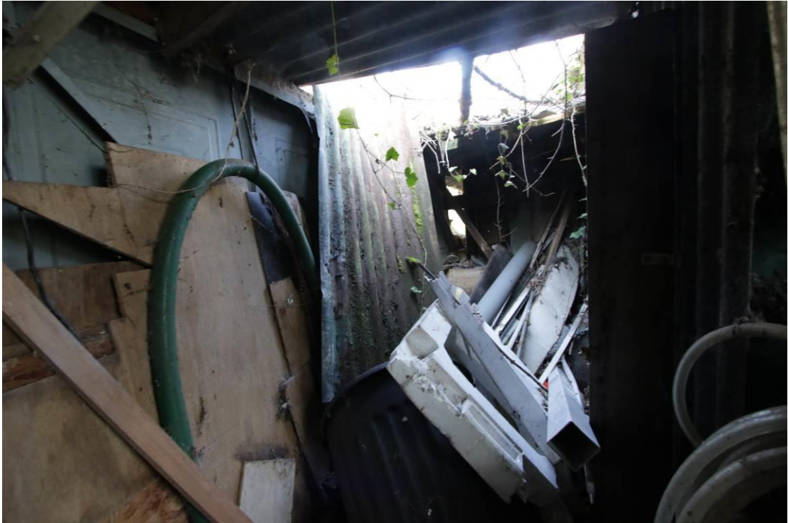
Photo 19: Access to all internal areas was not possible due to amount of materials stored in the sheds. A small amount of roofing was collapsed on a lean to to one of the shed sections
