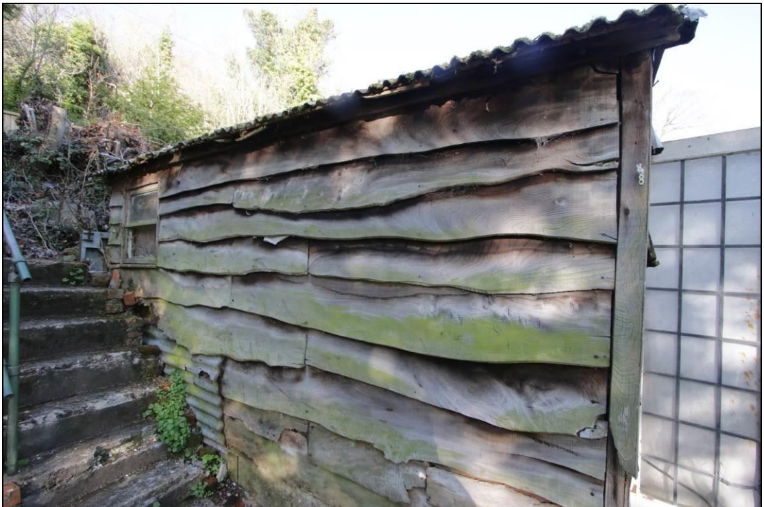
Photo 20: Cladding on sheds contained some higher potential gaps from warped wood.
