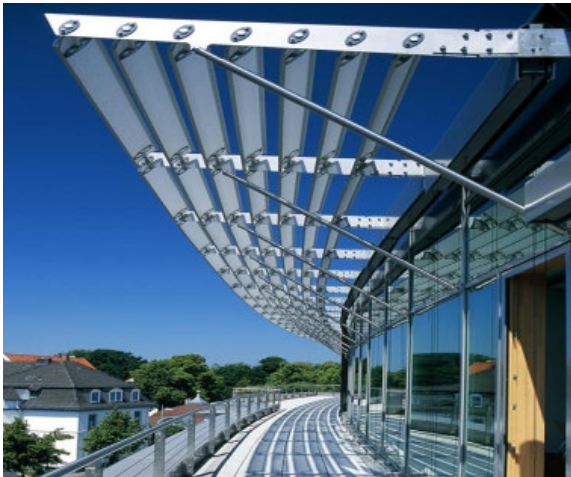
Figure 5 - Solar PV Louvres on the South Facade
