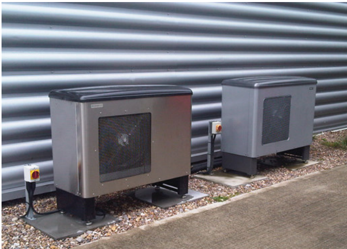
Figure 3 - Air Source Heat Pumps
