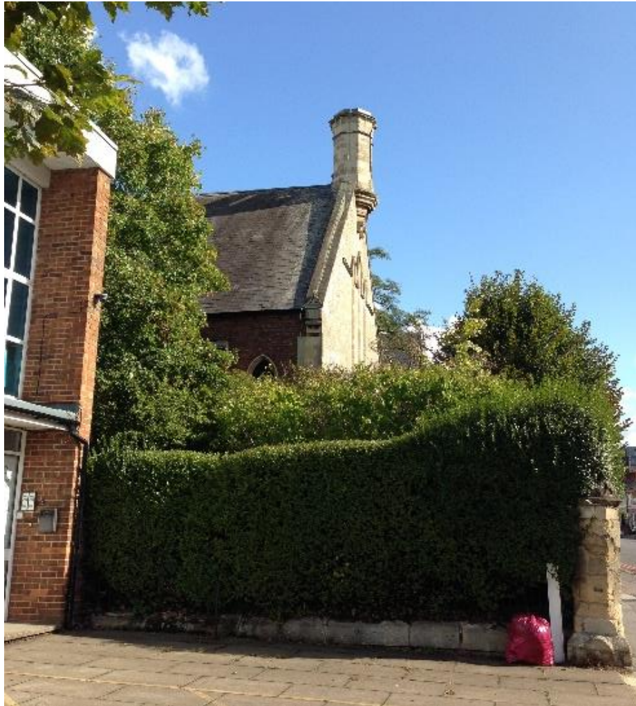
FIGURE 20 OVERGROWN HEDGE HIDES ORIGINAL PIER AND RAILINGS GA
