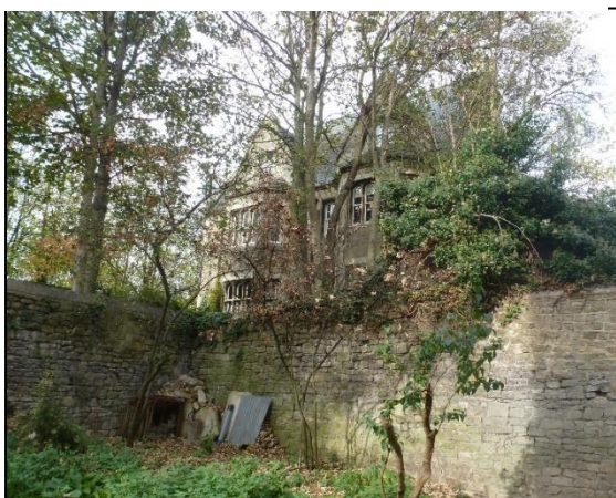
FIGURE 16 CARLISLE HOUSE SEEN BEYOND THE DAMAGED WALL CAUSED BY SELF-SEEDED SYCAMORE TREES
