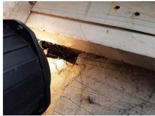
Photo 12: Image showing a gap between the breeze blocks and the metal structure of the facilities building on the roof on B1. There are cobwebs surrounding the hole.
