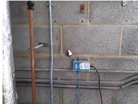
Photo 14: Image taken inside the facilities building on the roof of B2, showing a gap in the single-skin breeze blocks, allowing bats to potentially access the structure
