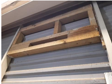
Photo 13: Image showing a wooden structure inside the facilities building on the roof of B2, which has gaps within it, providing opportunities for roosting bats
