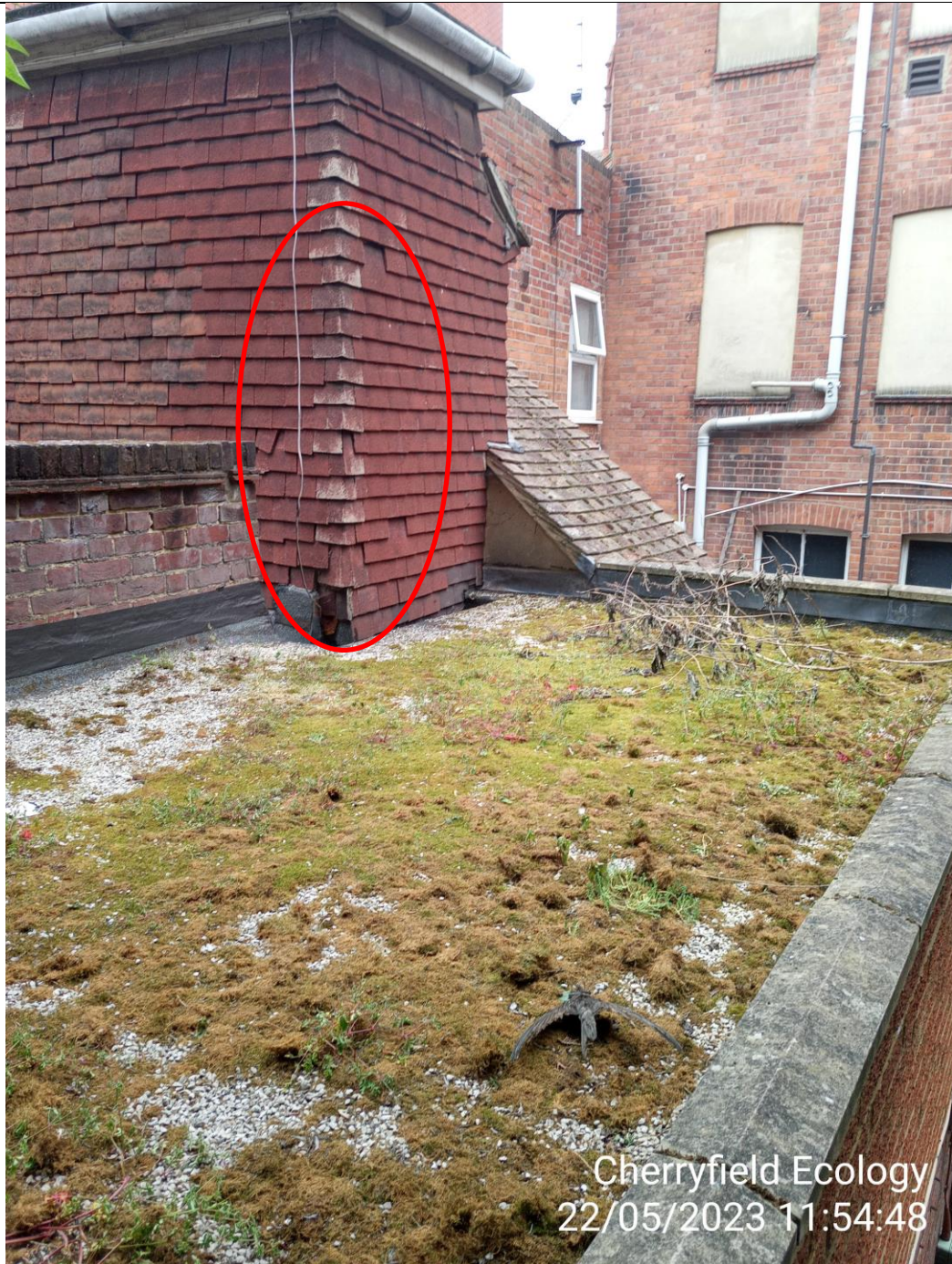
Figure 4: Example of lifted, broken and missing hanging tile with bat roost ptoential
