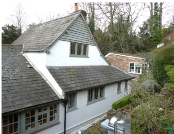
Figure 3: Rear elevation of 43A Church Road showing the lean-to that has been approved for removal and timber boards in the apex of the rear gable
