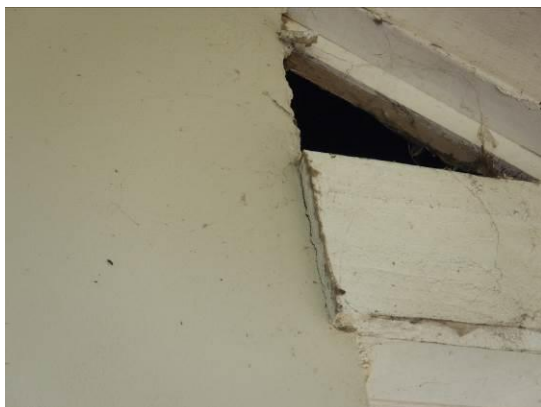
7. Small-sized bat dropping on northern elevation.
