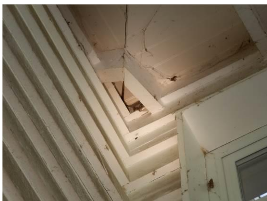
9. Active wasp nest in gap at eaves (eastern elevation).
