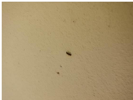
8. Small-sized bat dropping on northern elevation.
