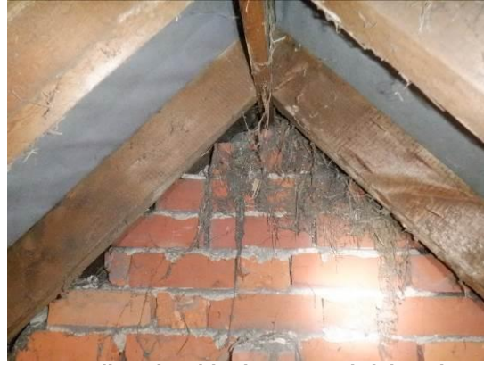
20. Heavily cobwebbed gap over brickwork gable (second roof void).
