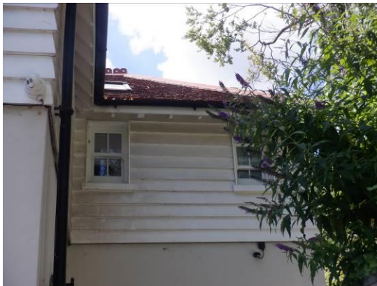
3. Uneven roof tiles.
