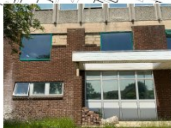
The existing buildings main facade is tired and dated; the building is in clear need of modernization and refurbishment to make the principal elevation more aesthetically pleasing
