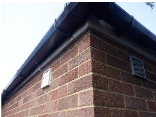
11. uPVC fascia tight to brickwork (south-eastern elevation).
