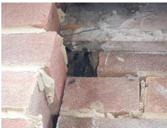
12. Cobwebbed gap in brickwork below soffit (south-eastern elevation).
