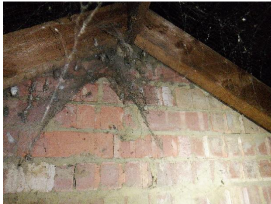
18. Cobwebbed brickwork gable (roof void).
