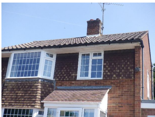
9. Occasional uneven hanging tiles (front elevation).
