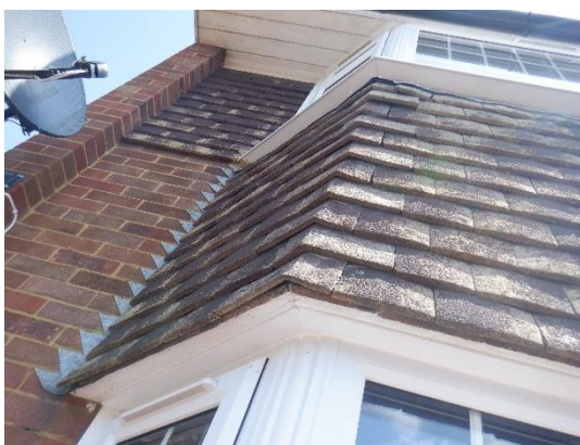
10. Lifted hanging tiles on bay window (front elevation).
