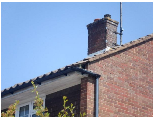
8. Damaged timber soffit at southern corner (northwest elevation).
