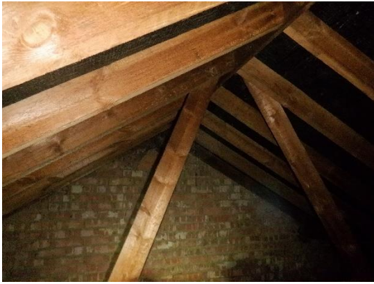
13. Cobwebbed ridge throughout (roof void).
