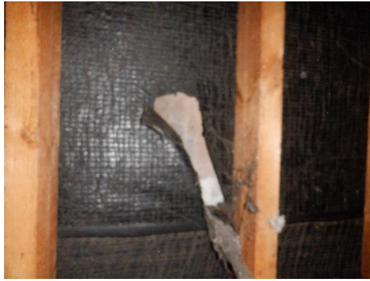
14. Large tear in bitumen roofing felt (roof void).
