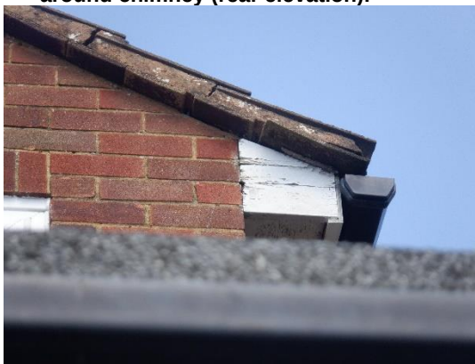
6. Small crack in verge mortar of limited extent (south-eastern elevation).
