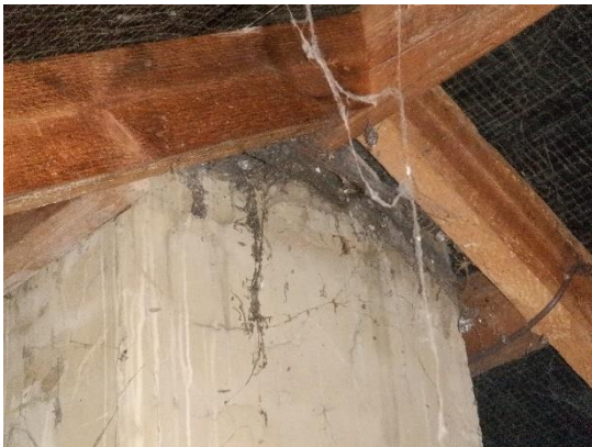
15. Heavily cobwebbed rendered chimney (roof void).
