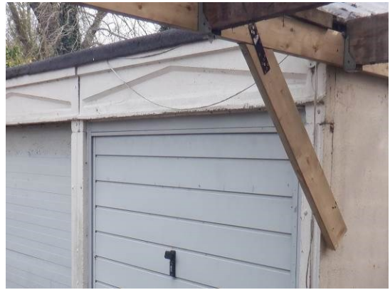
6. Frame tight to metal garage door (front elevation).
