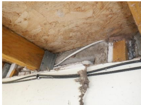
12. Gap in plasterboard ceiling with the underside of the boarded roof with fibreglass insulation visible.
