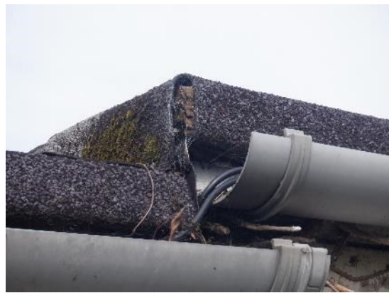
4. Superficial gap between the bitumen roofing felt and the barge board (rear elevation).
