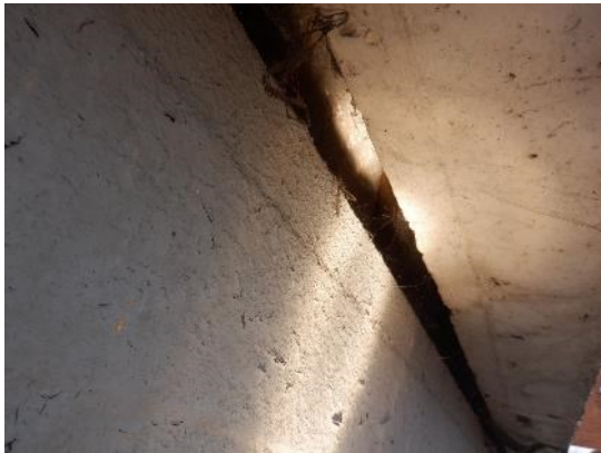
5. Large open gaps between soffit and concrete panels (front elevation).
