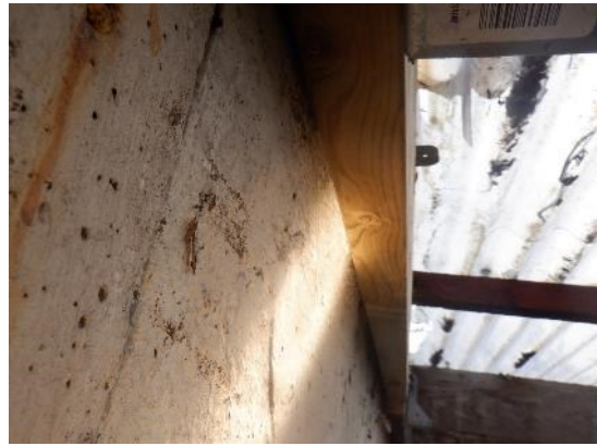
8. Open gap between timber frame and concrete wall (western elevation).
