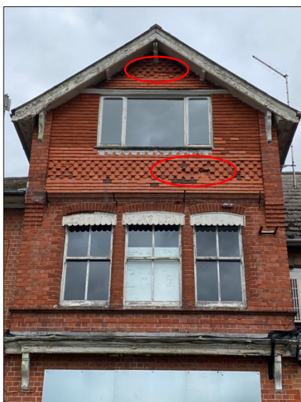
Photograph 15. Broken tile-hanging on rear gable
