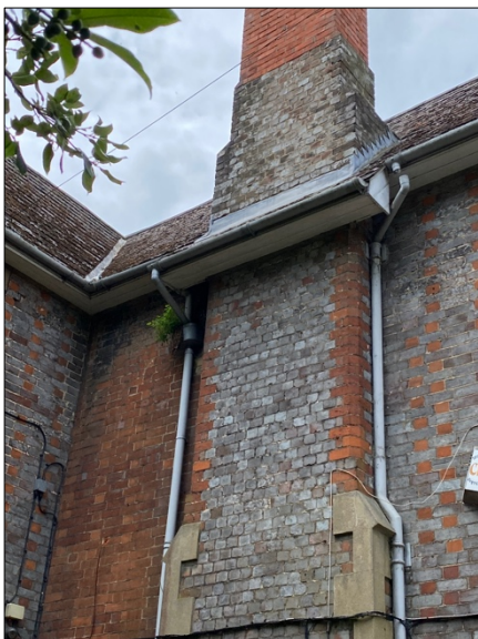
Photograph 13. Eastern elevation with gapped soffit
