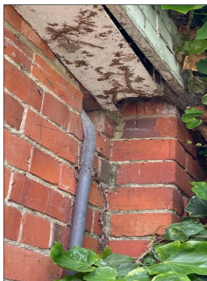
Photograph 16. Broken soffit on north-western garage
