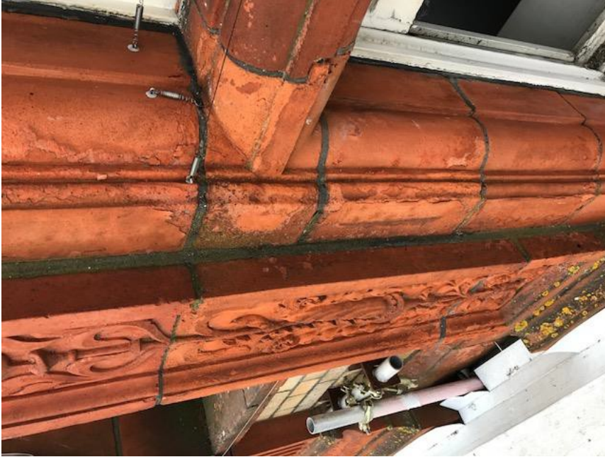
Cement pointing causing failure of the terracotta.
