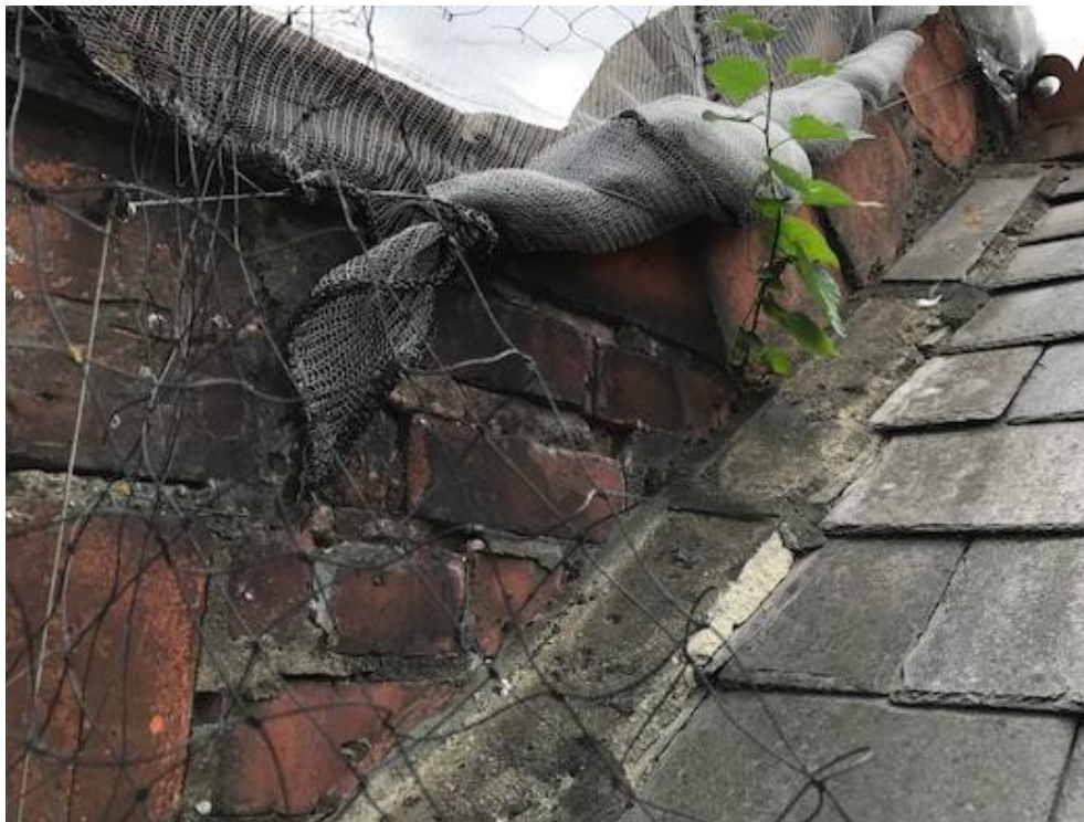
Cement pointing to failed brickwork supporting small gable.
