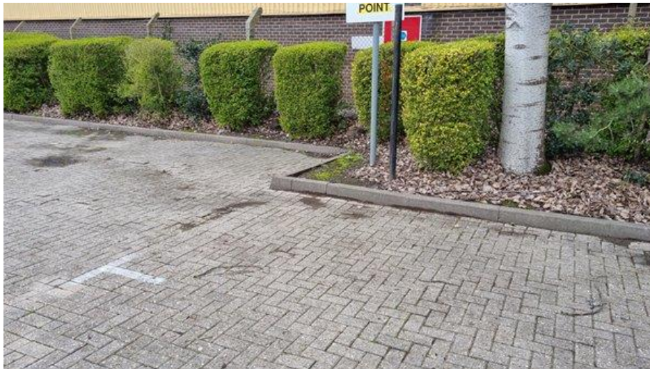
(Photo 3) base of T8 example of damage and disturbance to car park surface
