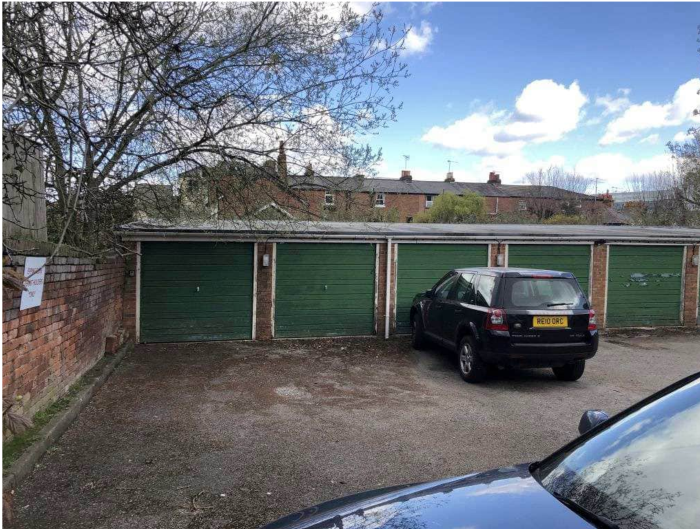
14. Photo showing a tree growing in adjacent property that is damaging the boundary wall. Future (additional) conflict with the adjacent wall can be forecast. Canopy oversails the existing garages.
