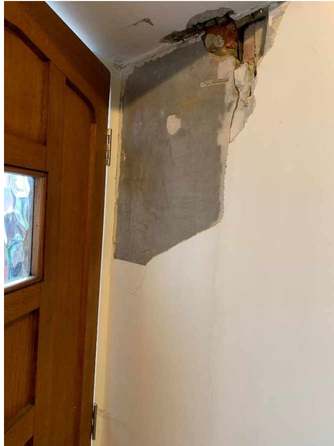
Figure 4 Dampness in hallway
