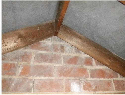
14. Small gaps behind rafters.
