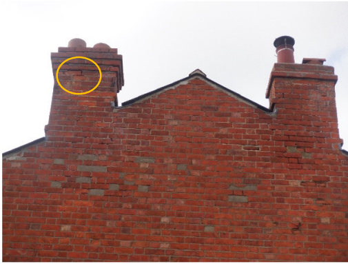
7. Gaps in chimney mortar, lead flashings flat.
