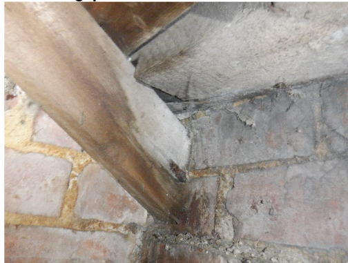
16. Small gaps behind rafters.
