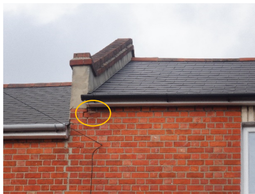
10. Gap in mortar near party wall.
