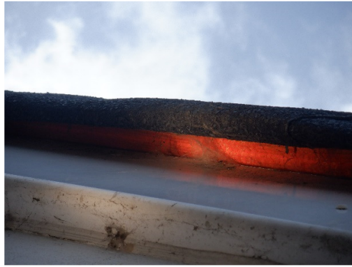
8. Gap under flat roof extension exposing space between roofing felt and uPVC barge board.
