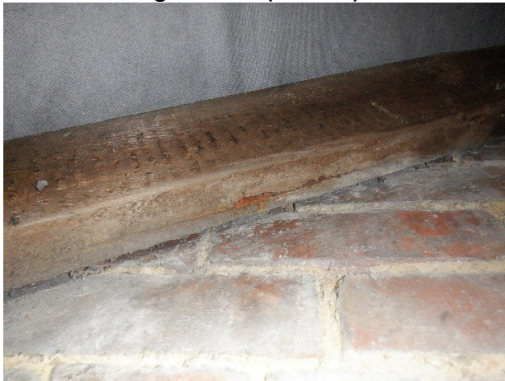
15. Small gaps behind rafters.
