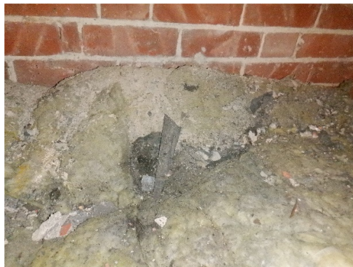
18. Very dusty fibreglass insulation throughout.
