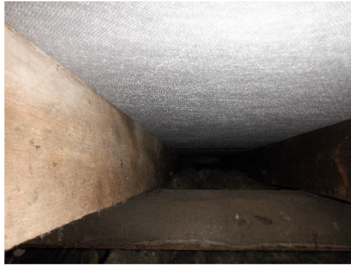
20. Eaves to soffits empty.
