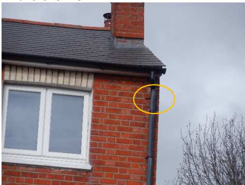
11. Gap in mortar near gable end.
