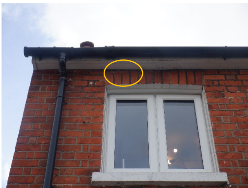
9. Small partly cobwebbed gap between soffit and brickwork.
