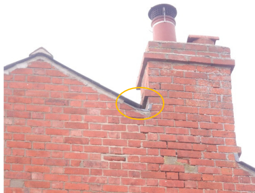
6. Large gap in gable verge mortar.
