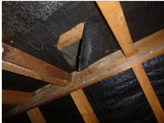
12. Tear in bitumen roofing felt (roof void).
