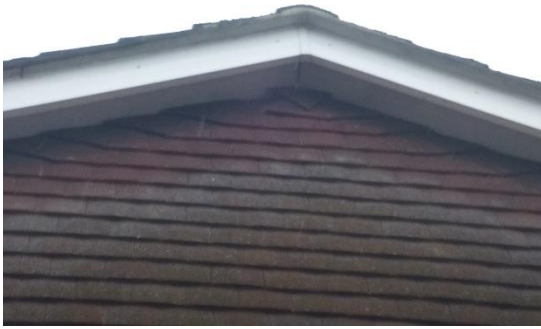
7. Slightly lifted hanging tile at front gable apex (front elevation).
