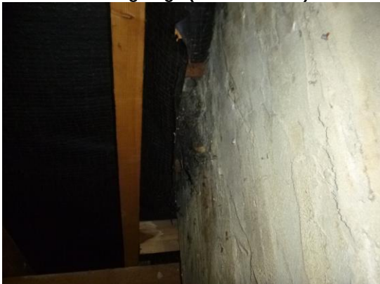
11. Cobwebbed gap in felt by chimney (roof void).
