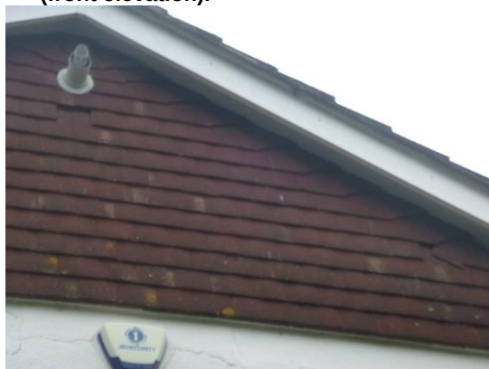
6. Missing and slipped hanging tiles on rear gable (rear elevation).
