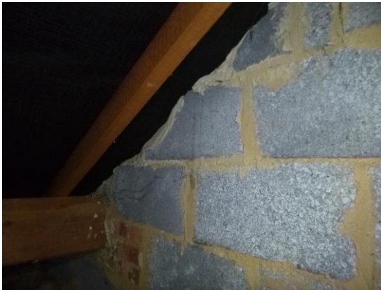
15. Mortar around edges of blockwork at rear gable end (roof void).
