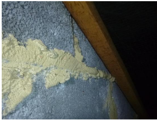
14. Blockwork tight to timber rafter at front gable end (roof void).
