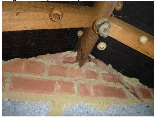
16. Small wasp nests at rear gable apex (roof void).
