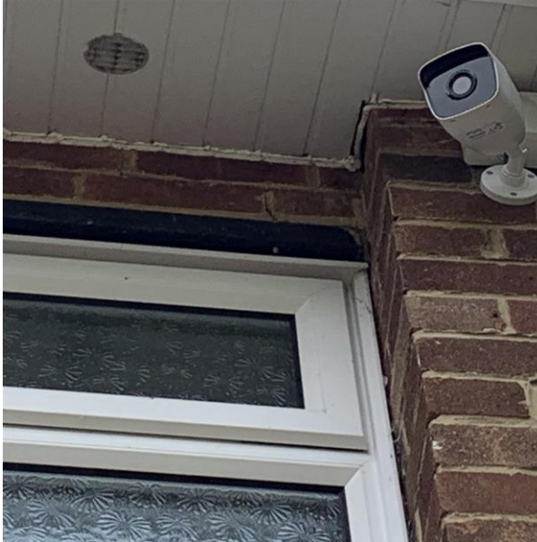
Crack above right bedroom window
