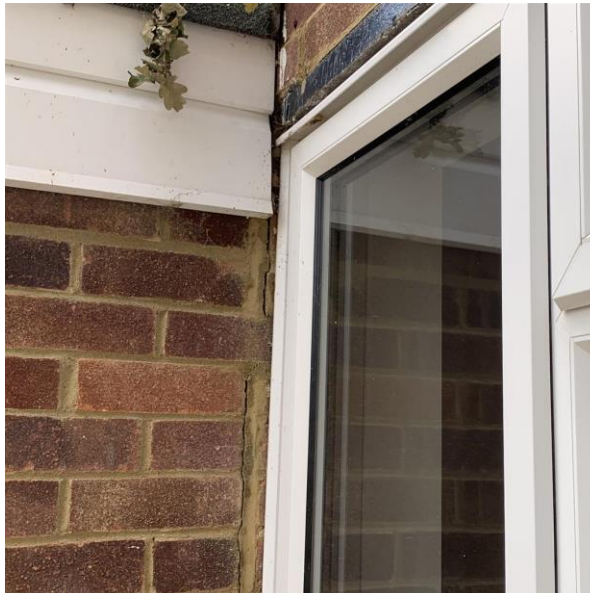
Porch junction crack - note previous repointing
