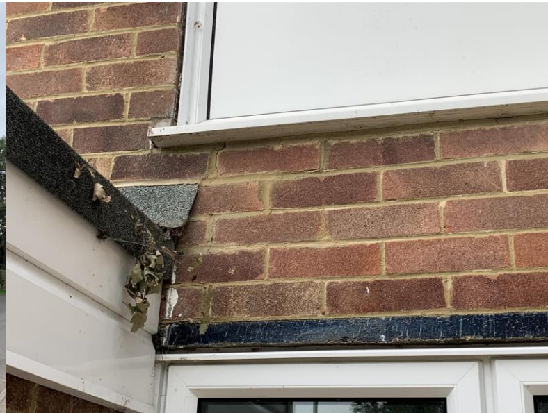
Crack below right bedroom window
