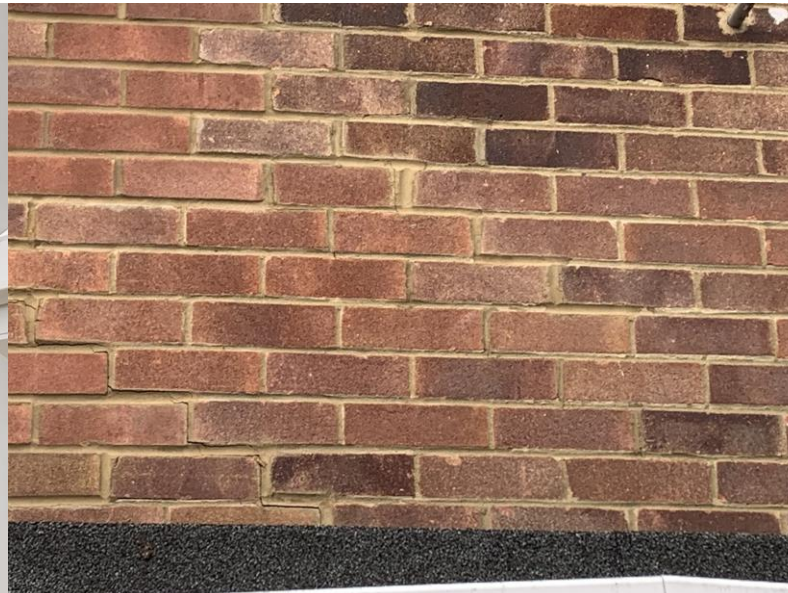
Stepped cracking on front elevation and previous repointing
