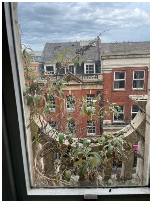
Image 7: Photograph showing how the lack of maintenance has resulted plants growing in the Station Road façade of the building.
