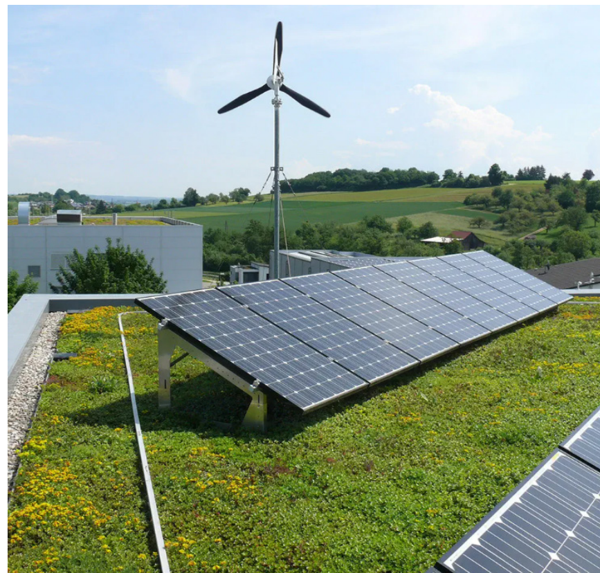
PHOTOVOLTAICS WITH BATTERY STORAGE ON FLAT ROOF
