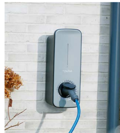
EV CHARGING POINT
